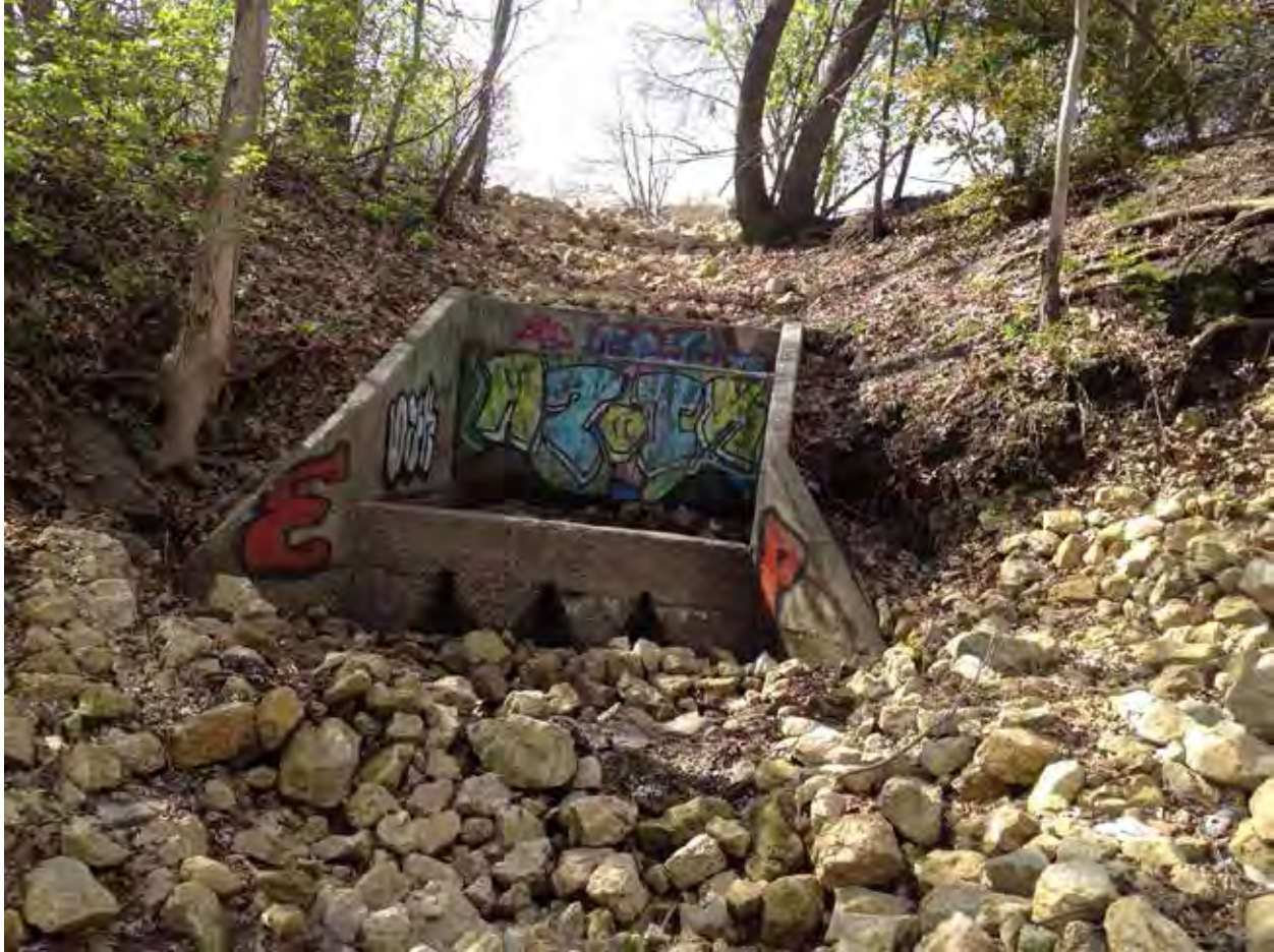
Photo 1-1 Energy dissipation structure downstream of the 27-inch outfall and erosion of adjacent side slope (May 2014 site visit)
