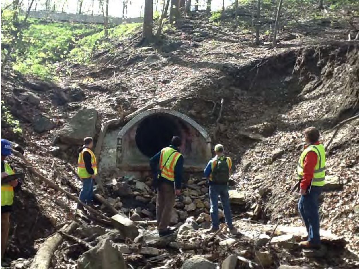
Photo 1-3 Erosion and scouring at the outfall of the Cherokee Heights culvert (May 2014 site visit)
