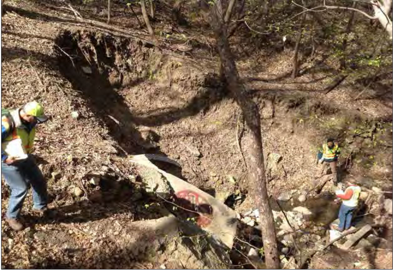
Photo 1-2 Erosion adjacent to the storm sewer outlet in Cherokee Heights ravine (May 2014 site visit)
