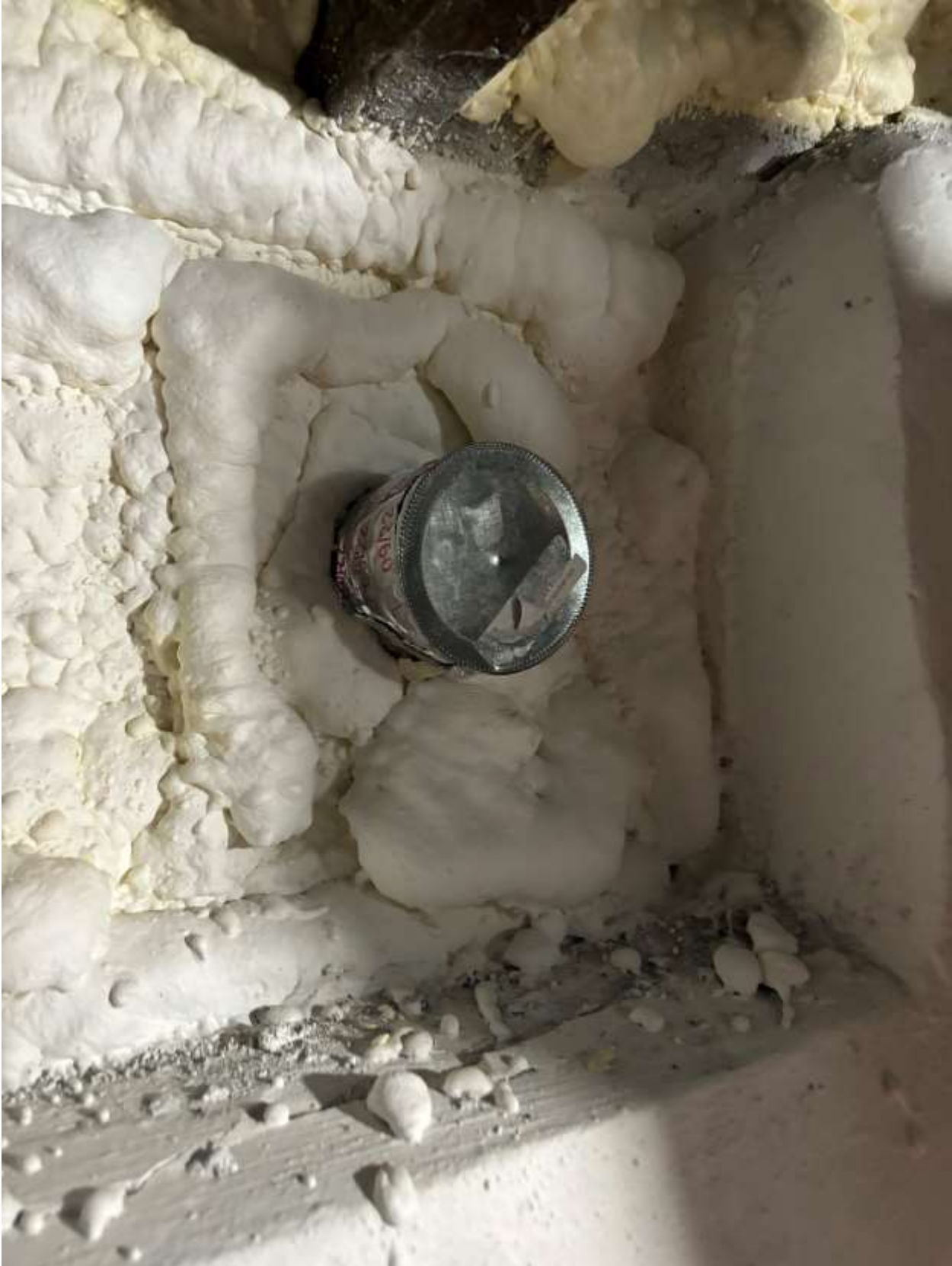
705 Magnolia Ave screen dryer vent
