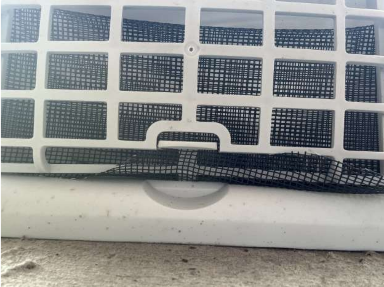
705 Magnolia Ave screen dryer vent
