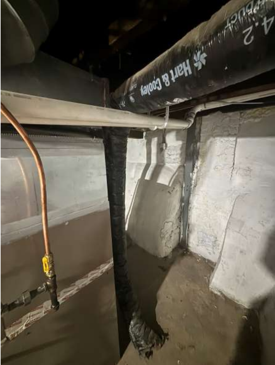
705 Magnolia Ave screen dryer vent
