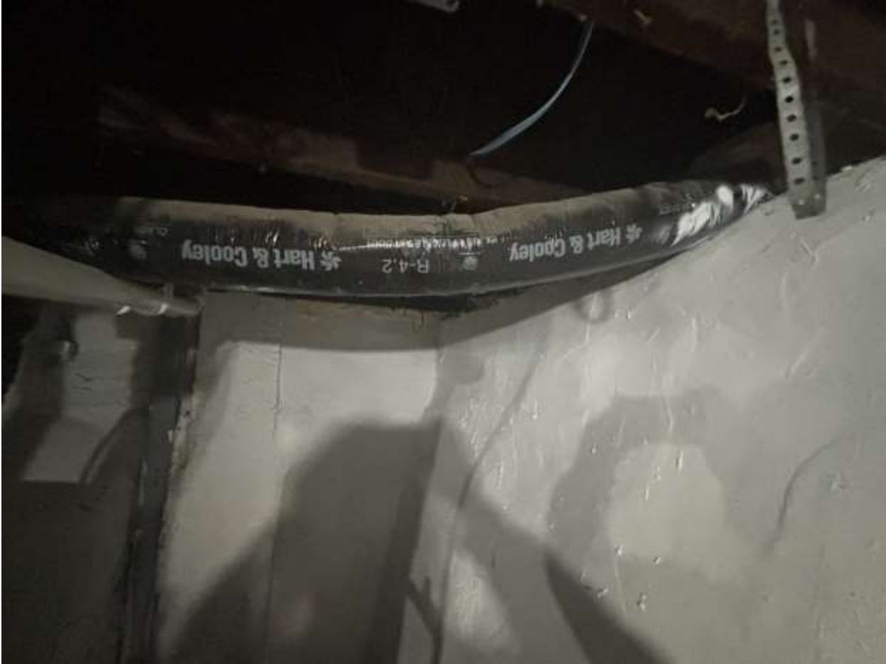
705 Magnolia Ave screen dryer vent
