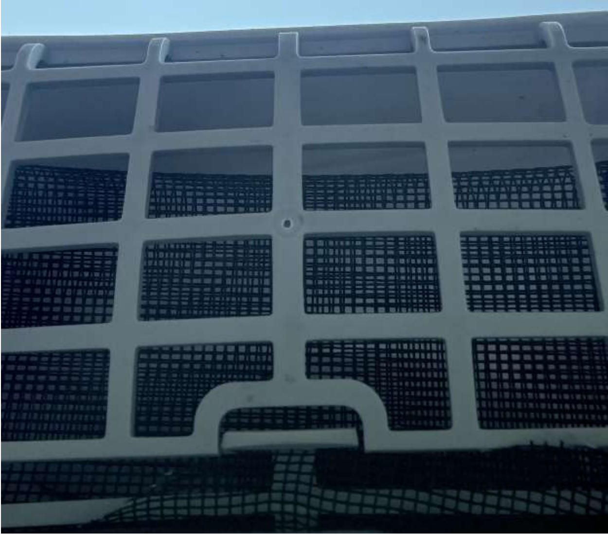
705 Magnolia Ave screen dryer vent
