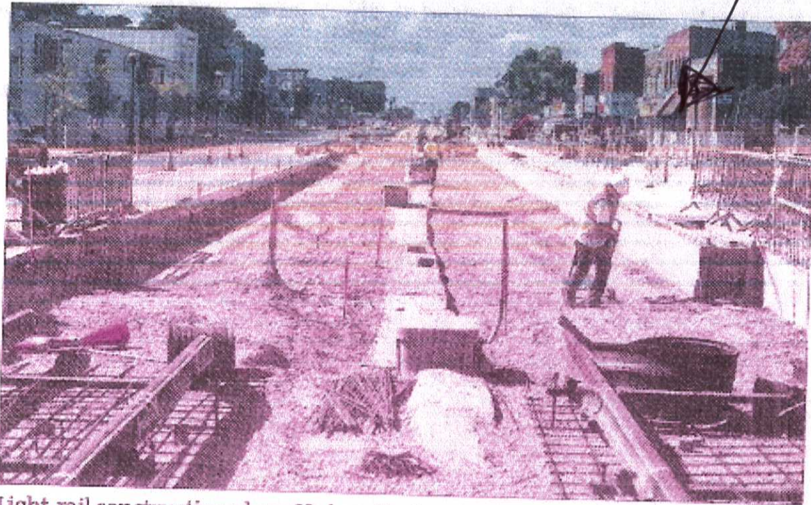
Light-rail construction along University Avenue in St. Paul has made conditions very difficult for the businesses there.
