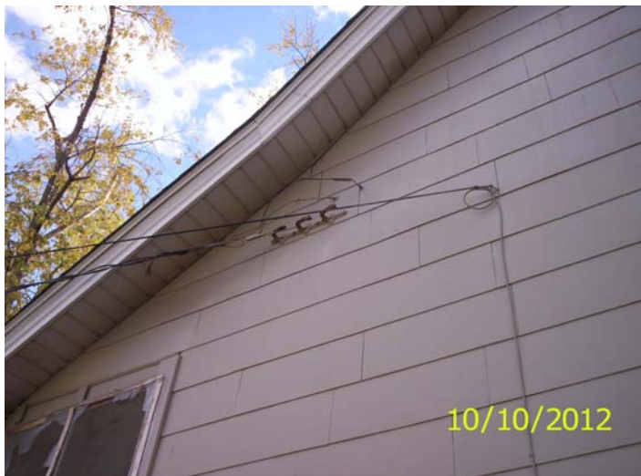
2-conductor knob & tube electrical service drop
