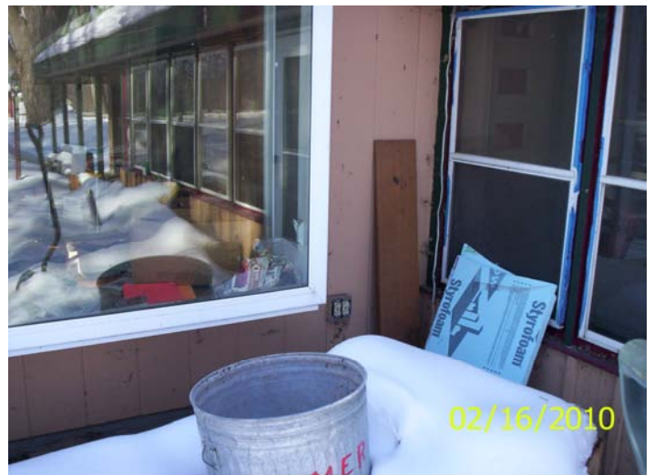
Open electrical outlet
