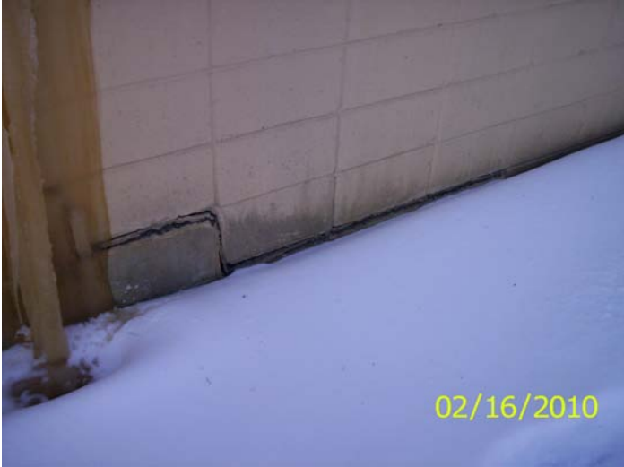
Large separating shifting crack
