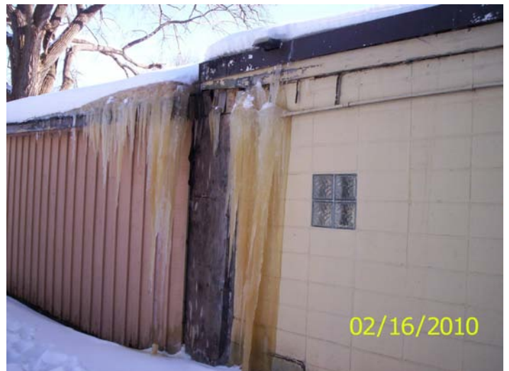
Rotted eaves house and garage, rotted wall
