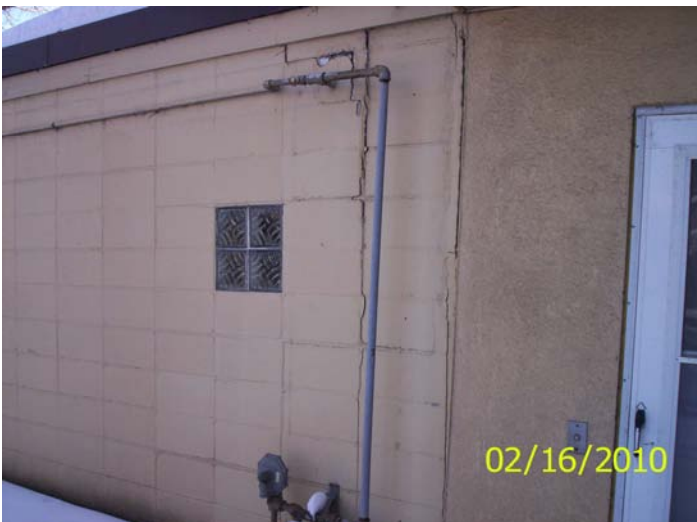
Large separating crack
