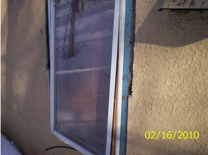
Unfinished window installation, boarded on interior
