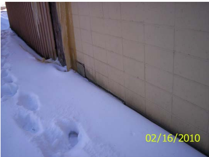
Large separating shifting crack
