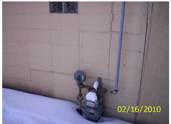
Cracking in masonry
