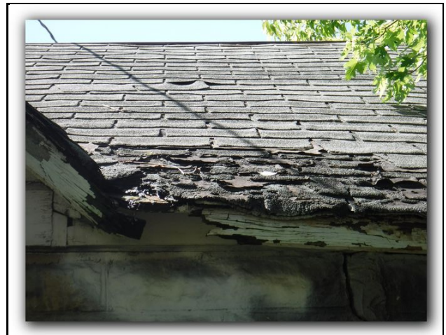
8 Roof in poor condition. Contributing to water intrusion and rot of roof/attic framing.
