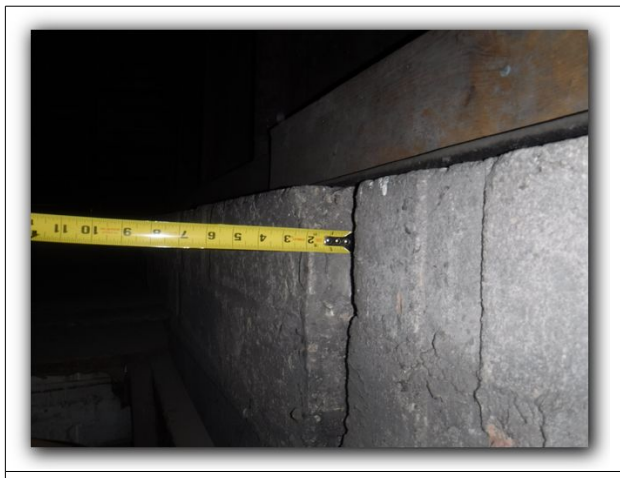
9 NW corner. Cracked and displaced. Consider repairs.
