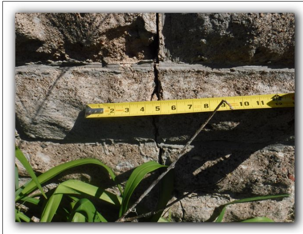
5 Vertical crack in CMU wall. Seal to prevent water intrusion.
