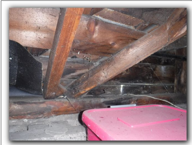
15 Attic framing - including ceiling joists, roof joists and collar ties in fair condition.
