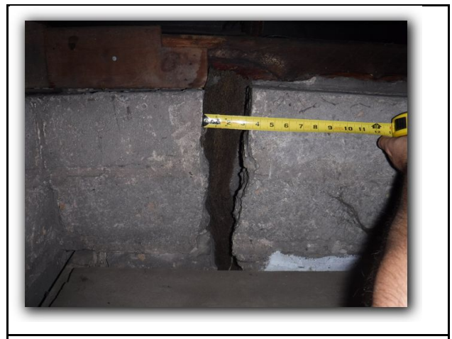
10 No recent movement reported. Monitor for movement if not proceeding with repairs.
