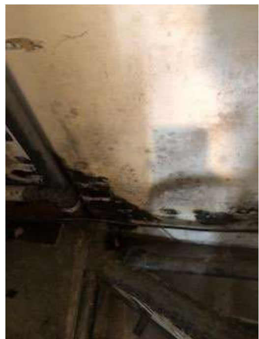
20: Mold at laundry room walls
