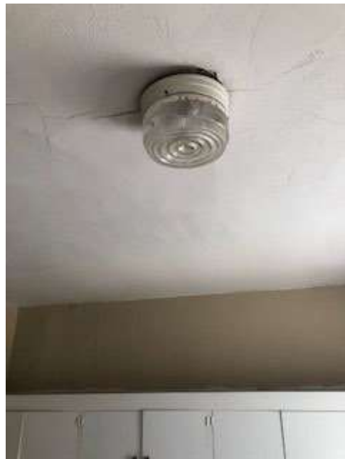
28: Cracking near light fixture in tenant unit
