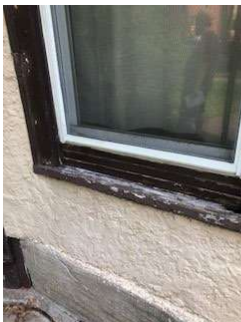
3: Rotting/peeling exterior trim
