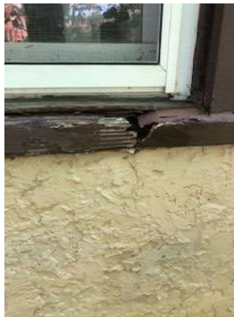
4: Rotting/peeling exterior trim and cavity
