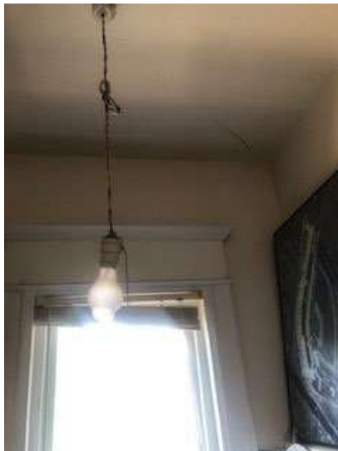
45: Light in tenant unit w/o cover
