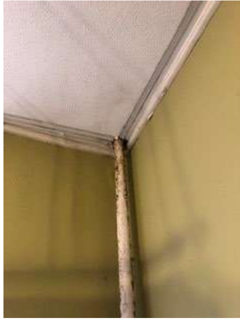
26: Mold/rust on exposed pipe
