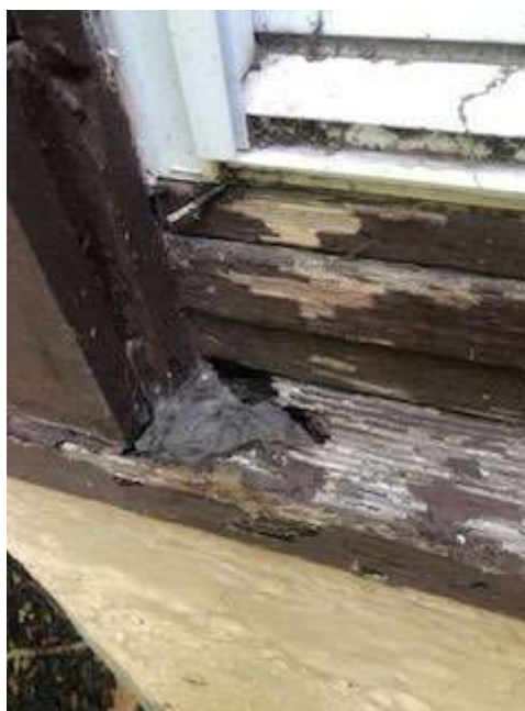
2: Rotting/peeling exterior trim and cavity
