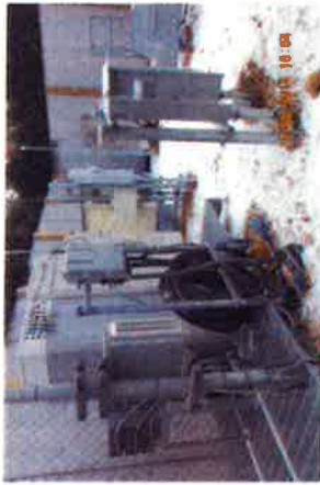
EXISTING T-MOBILE EQUIPMENT
