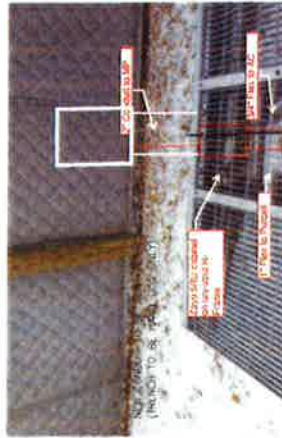
NEW ZAYO CABINET LOCATION
