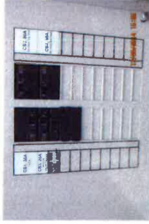
EXISTING T-MOBILE AC PANEL
