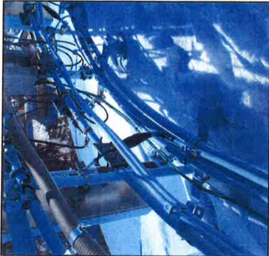
2 COAX ON TOWER SCALE: NONE
