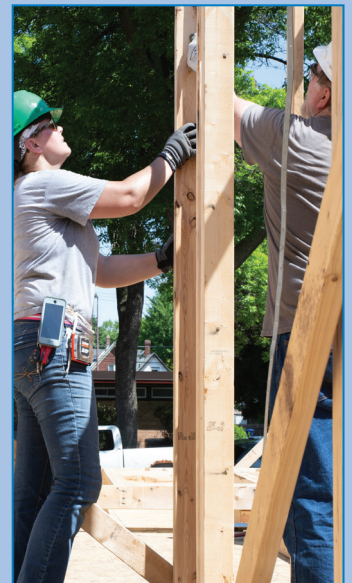
Above right, Hayley Heidelberg, (left) emergency management and security supervisor, and Bryan Jensen, welder, work on framing up an internal wall at the home being built at 722 LaFond Ave. in Saint Paul. Every year, volunteers from the city take part in a Habitat for Humanity build. The water utility shared the day with staff from the Department of Safety and Inspections, human resources, and the mayor's office.
