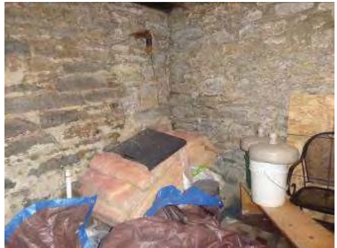
28. Pipes in basement of 625 University Avenue West
