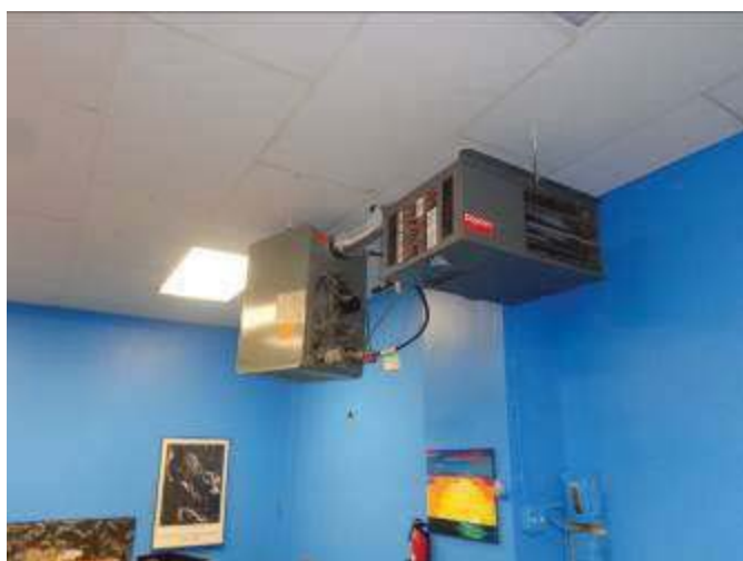
23. Ceiling-mounted natural gas-fired heater in the 631 University Ave W tenant space
