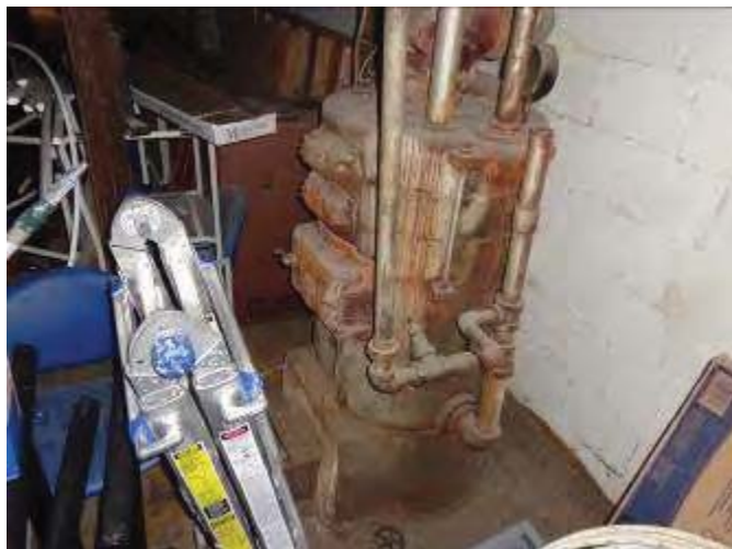
21. Old/former boiler in basement of 629 University Ave W
