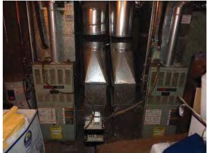
26. Furnace in basement of 625 University Avenue West
