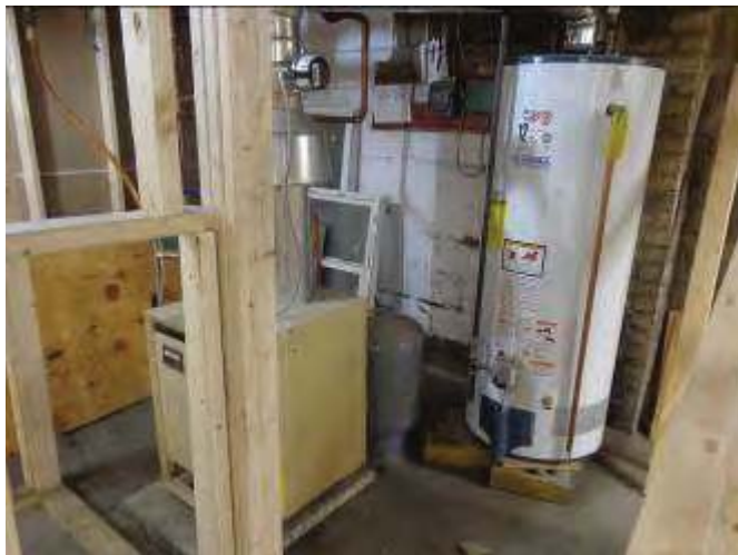
20. Boiler and water heater in basement of 629 University Ave W
