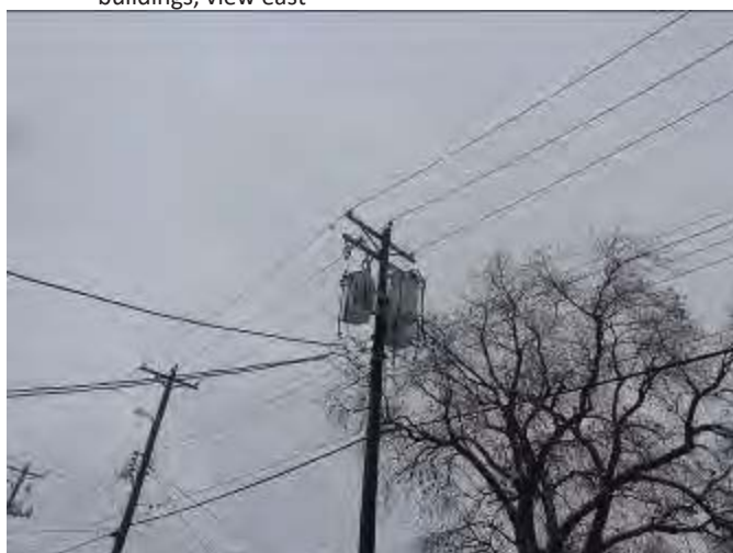
11. Pole-mounted transformers in the alley which bisects the Property
