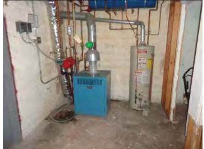
14. Boiler and water heater in the basement of the 633 University Ave W building
