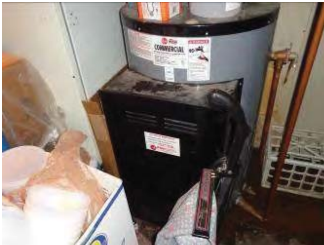
27. Water heater in basement of 625 University Avenue West
