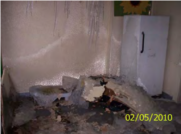
Kitchen, ice covered appliance, wall, floor
