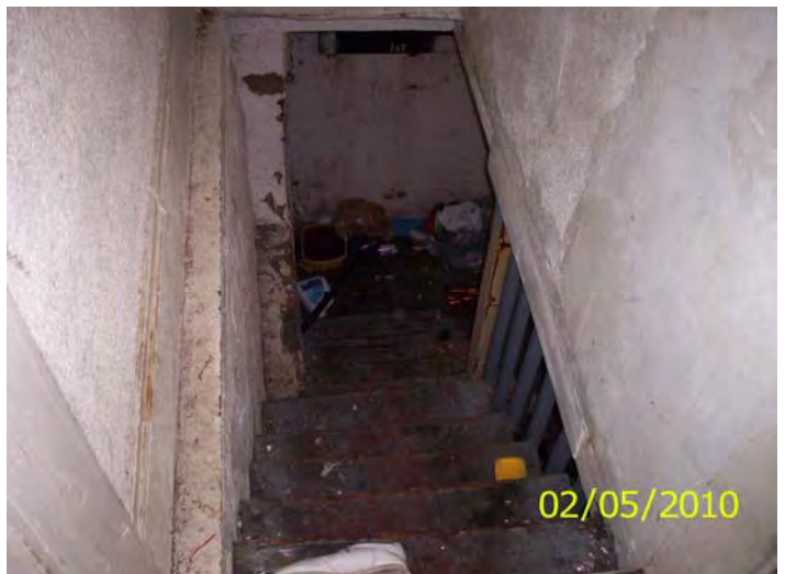
Stair way to basement, flooding, no hand rail
