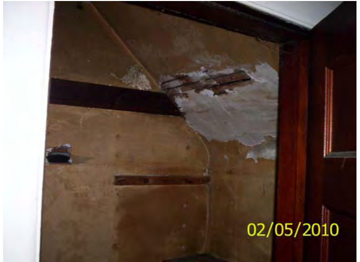
Damaged ceiling 2 nd floor bathroom
