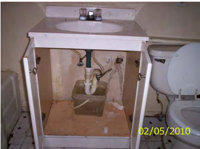
Improper trap repair, leaking
