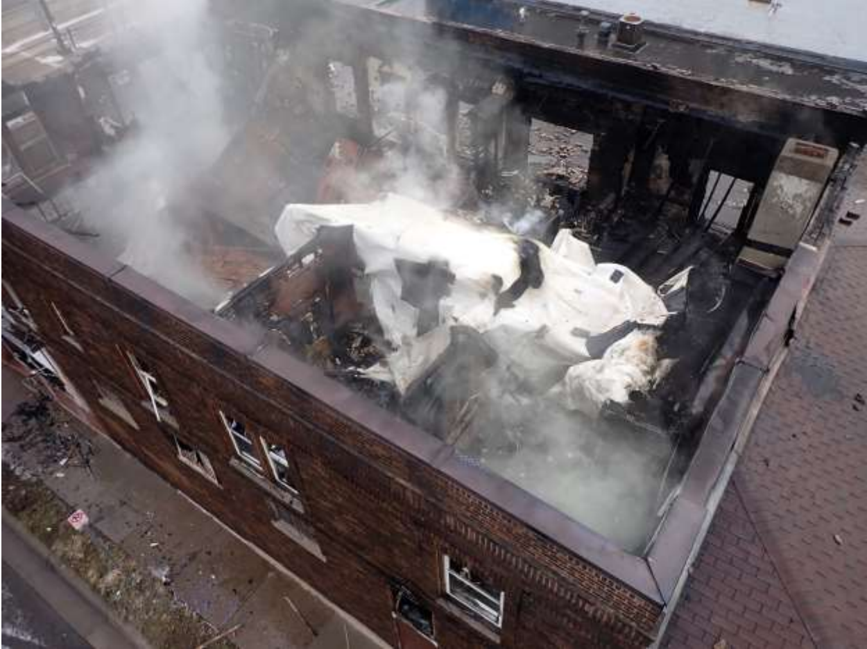
916-918 University Ave W.Fire Photos 1-10-24
