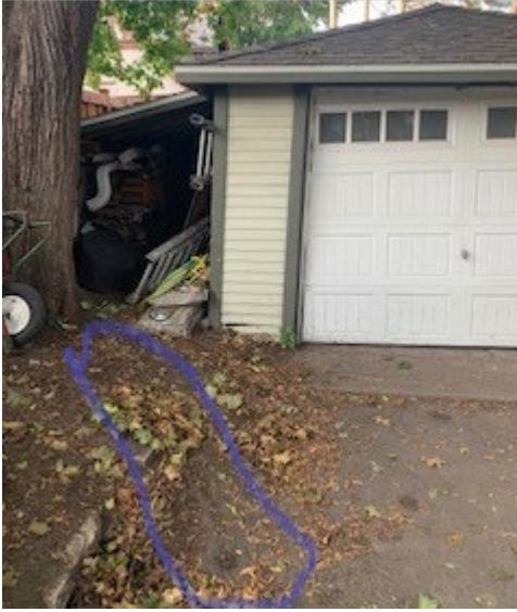
Old growth tree with root growing over driveway (and other roots under foundation causing foundation to buckle.
