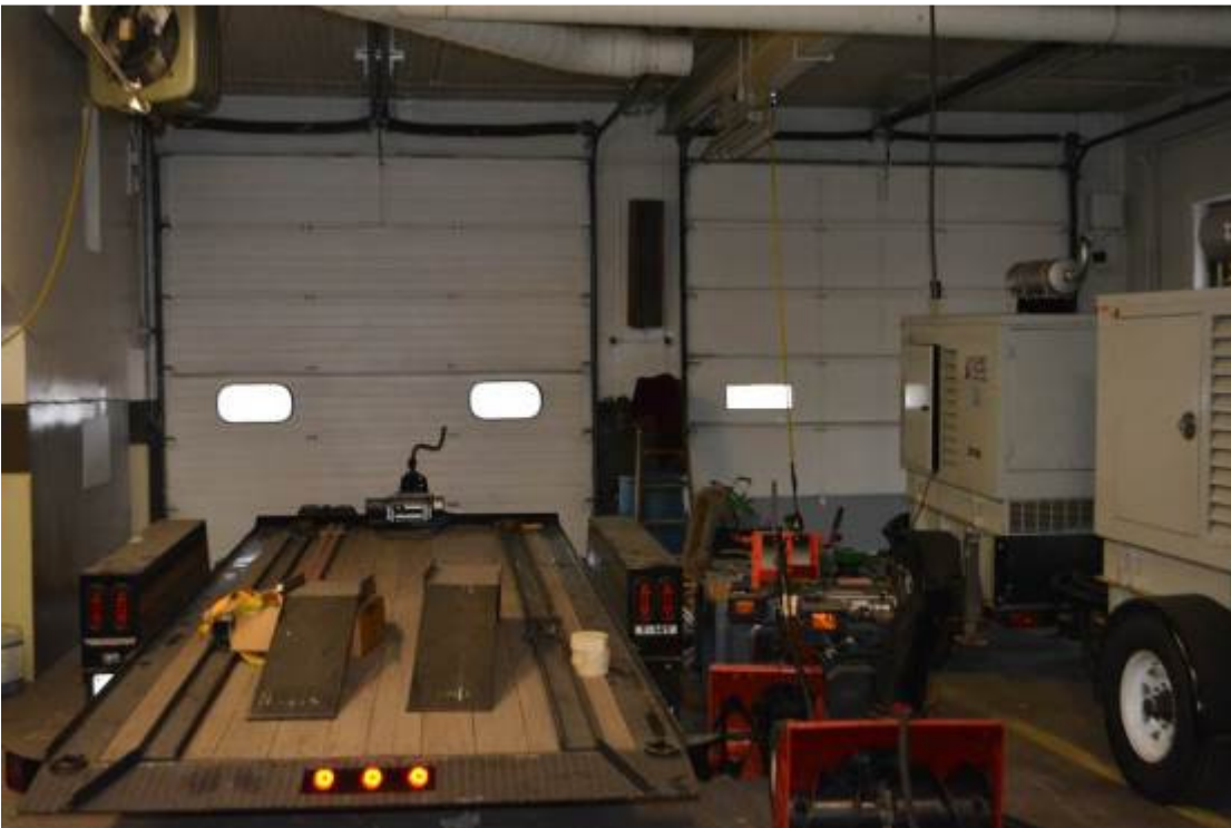
Photograph 8. Interior of apparatus bay in original 1885 portion of building, camera facing north.
