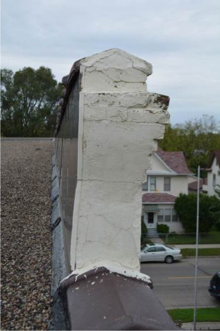
Photograph 5. Parapet of original portion of building. Photograph shows the addition of a parapet cap to match the detailing of the 1911 addition.
