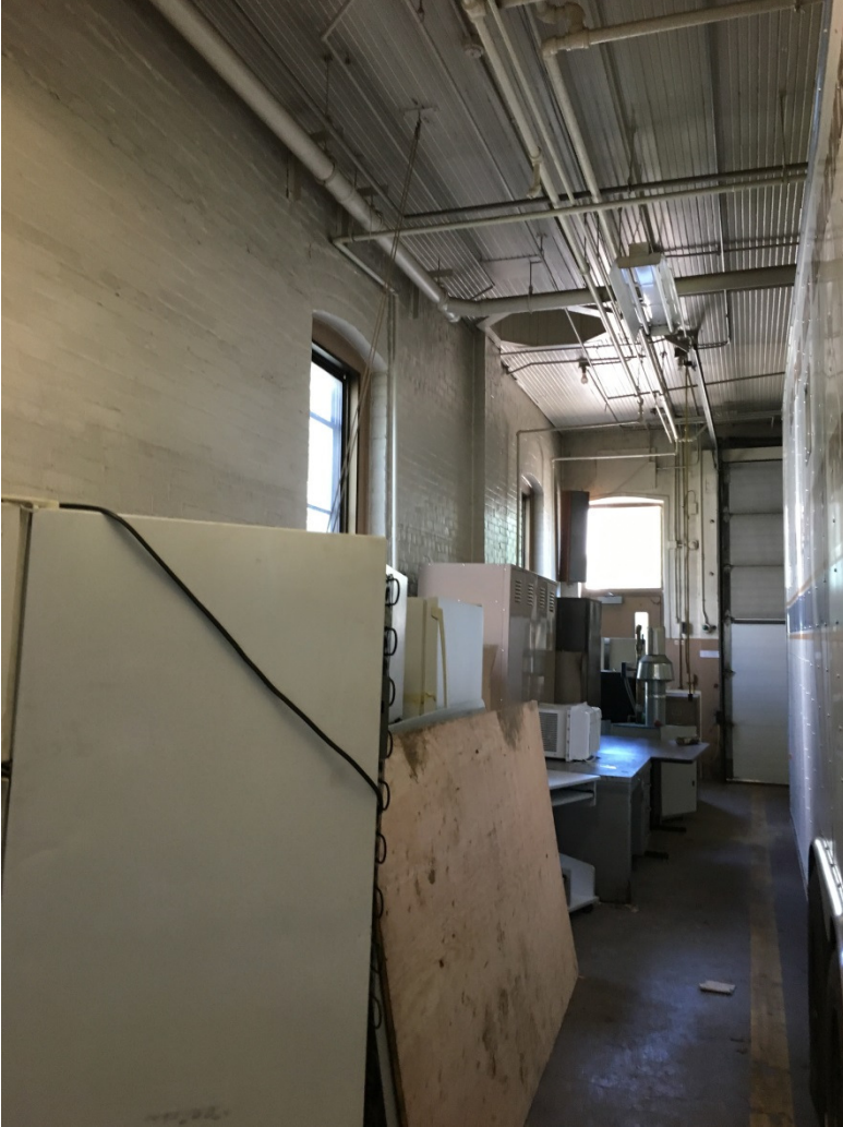
Photograph 16. North fire pole opening, photograph facing north, taken from 1911 apparatus bay. (photograph by HPC Staff June 30, 2017)
