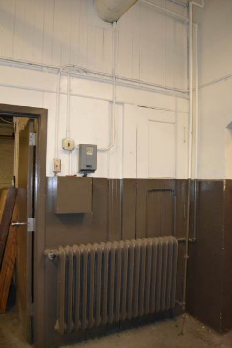
Photograph 11. Door to hose tower, blocked by radiator. Camera facing south.
