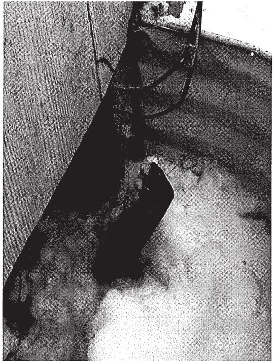
Photo 4 – Window Well with High Interior Grade Level
