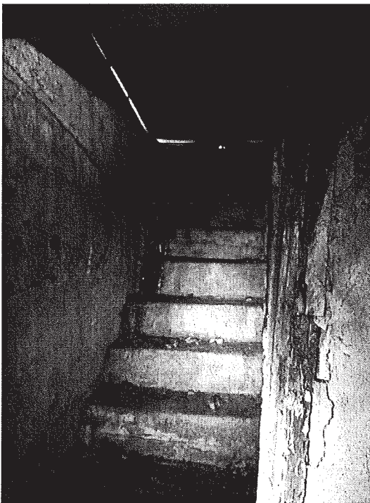
Photo 7 – Stair Access Allowing Moisture Infiltration
