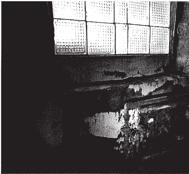
Photo 5 – Low Window Sill Allowing Moisture Infiltration
