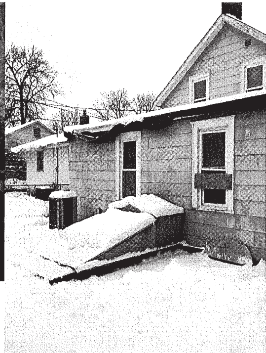
Photo 6 – Uninsulated, Unprotected Exterior Stair Access
