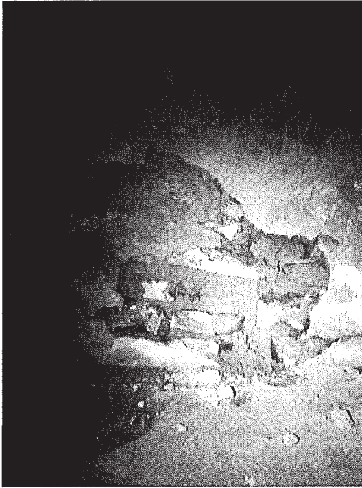
Photo 9 – Damaged Parge Coat and Crumbling Foundation Wall
