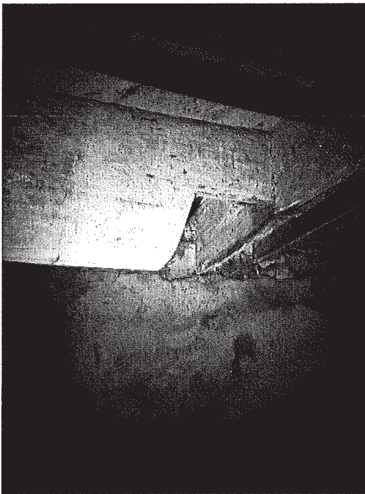
Photo 11 – Notched Floor Joist without Joist Hanger
