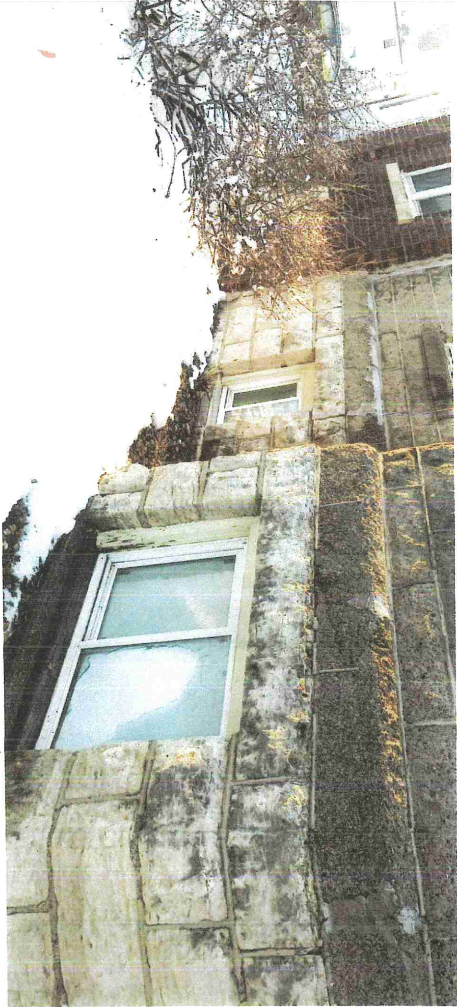
474 Herschel South window unrepaired for several weeks Picture taken 4/1/2022
