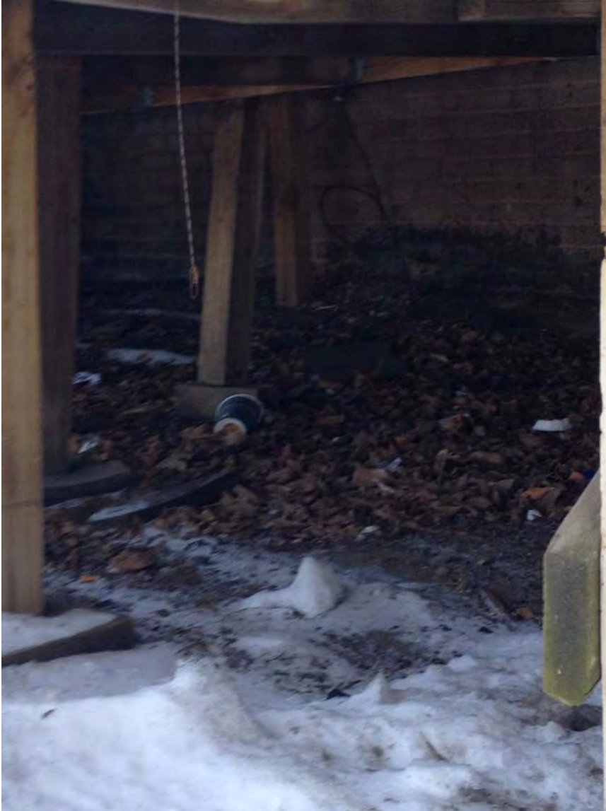
Enlargement showing one structural member out of plumb.
