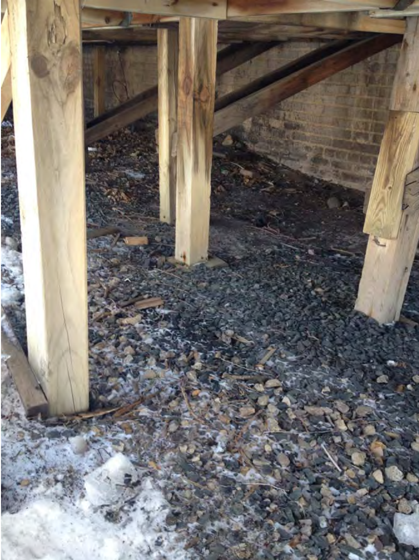
Structural elements of exterior loading dock which also serves as a means of egress from the building.
