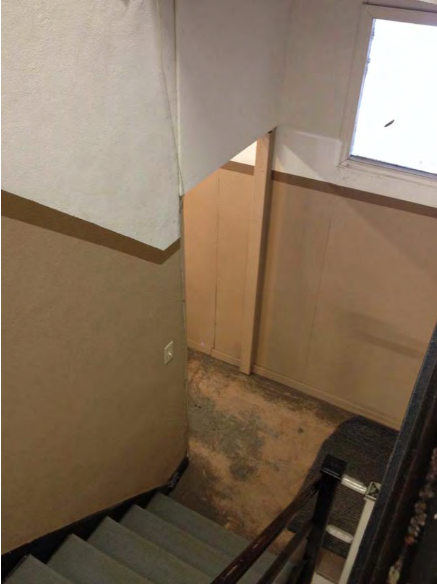
Opening at 2 nd floor. No door but a landing on both sides of the opening.
