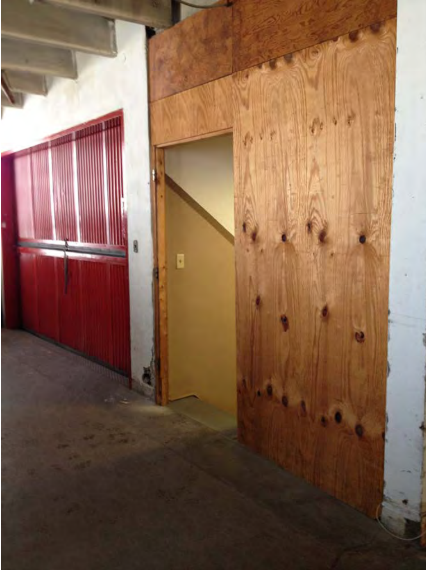
Opening at the 3 rd floor. No door but evidence of a past plywood door and hasp locking arrangement. No landing on stair side where door opening is.
