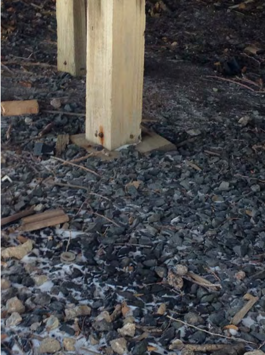
Enlargement showing the lack of footing.
