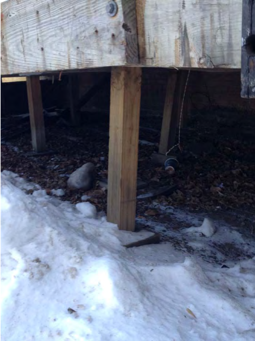
Structural elements of exterior loading dock which also serves as a means of egress from the building.
