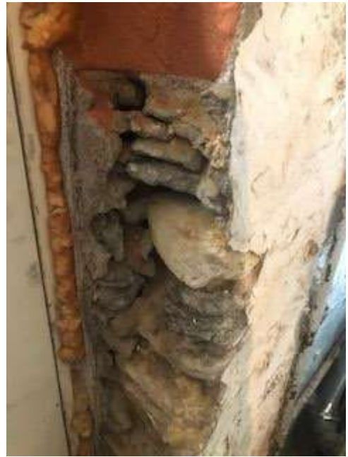
11: Settling foundation with holes
