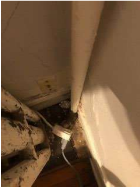
32: Missing flooring in tenant unit
