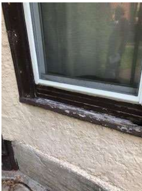
3: Rotting/peeling exterior trim
