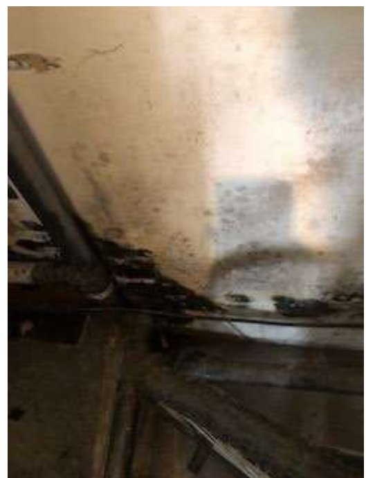
20: Mold at laundry room walls
