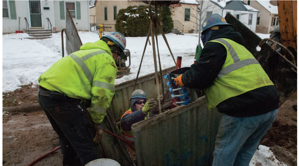
Joe Garcia, water system worker (center) receives a sleeve from Gordon Carney, water utility worker, (right, back to camera) while Jeremy Kiecker, water utility worker, looks on. Dustin Schluessler, water system worker, was in the box, working on the main break. The crew was at 1471 North Maywood on January 16. Brian Gomez was the crew foreman with Tom Lanigan at HEO and Rich Reeves operating the truck.
