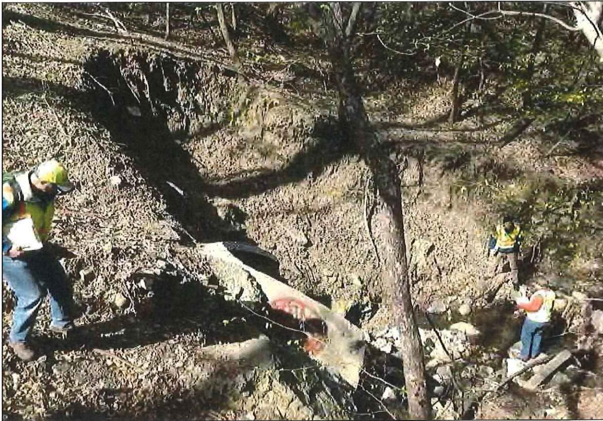
Photo 1-2 Erosion adjacent to the storm sewer outlet in Cherokee Heights ravine (May 2014 site visit)
