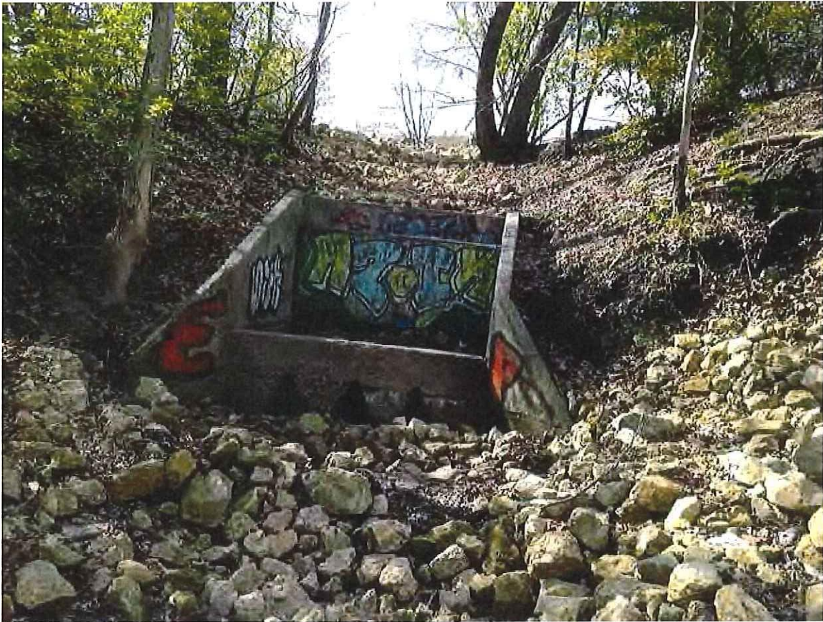
Photo 1-1 Energy dissipation structure downstream of the 27-inch outfall and erosion of adjacent side slope (May 2014 site visit)
