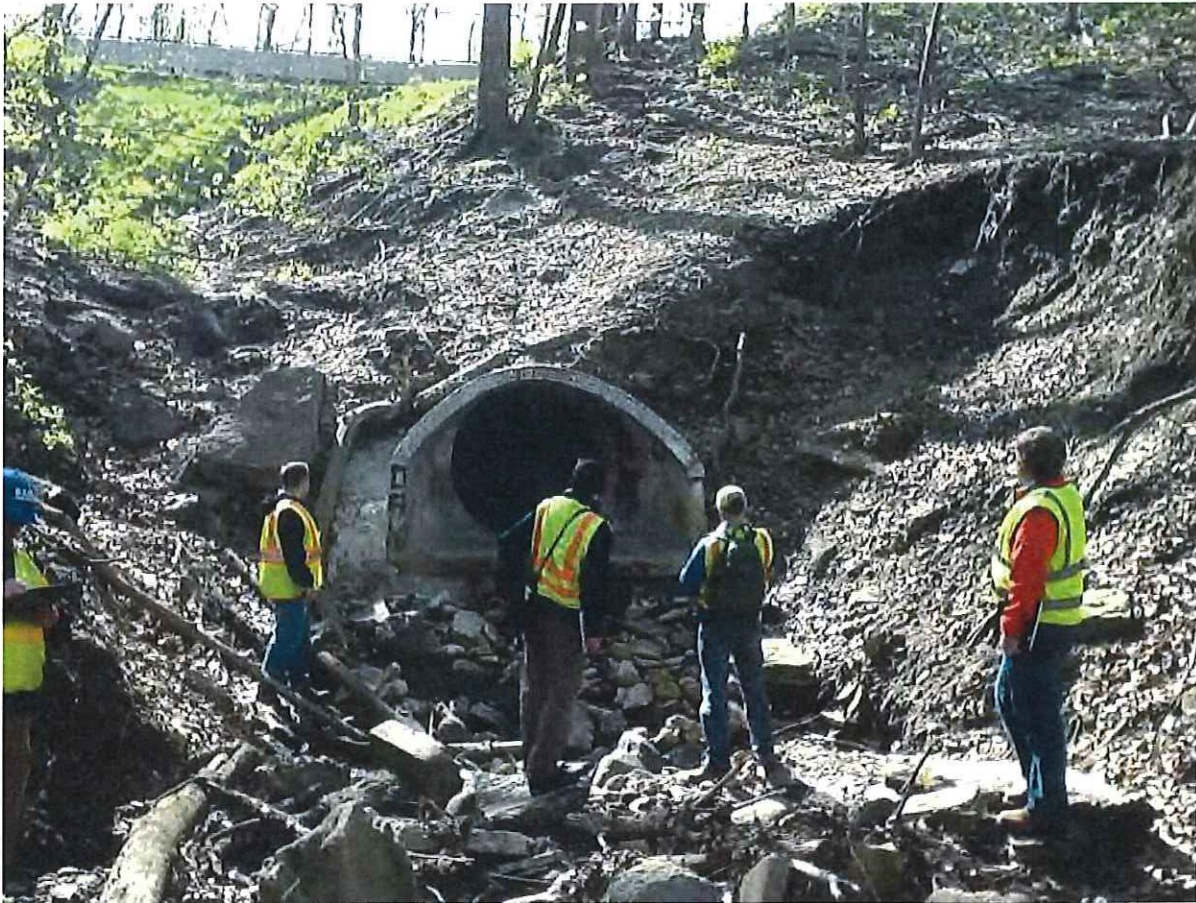
Photo 1-3 Erosion and scouring at the outfall of the Cherokee Heights culvert (May 2014 site visit)
