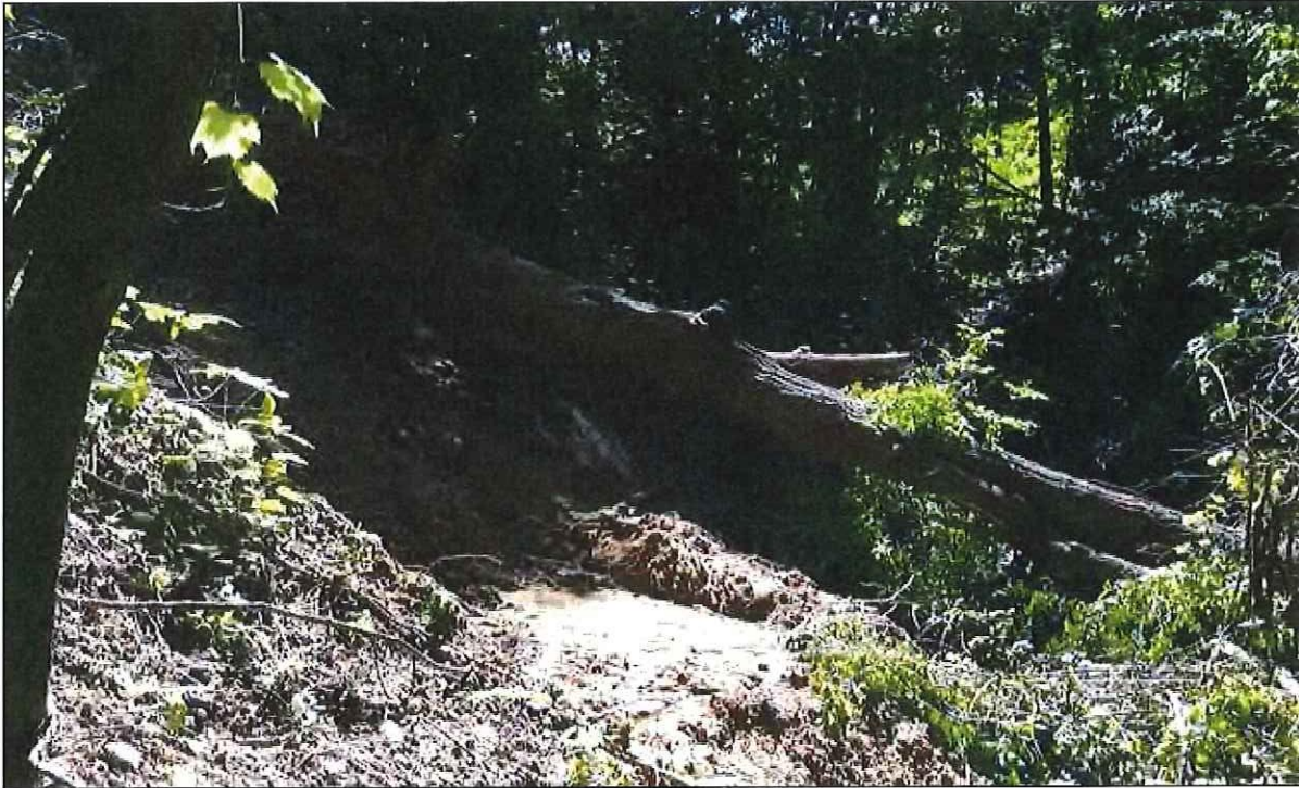
Photo 1-4 Cherokee Heights ravine slope failure (July 2014 site visit)
