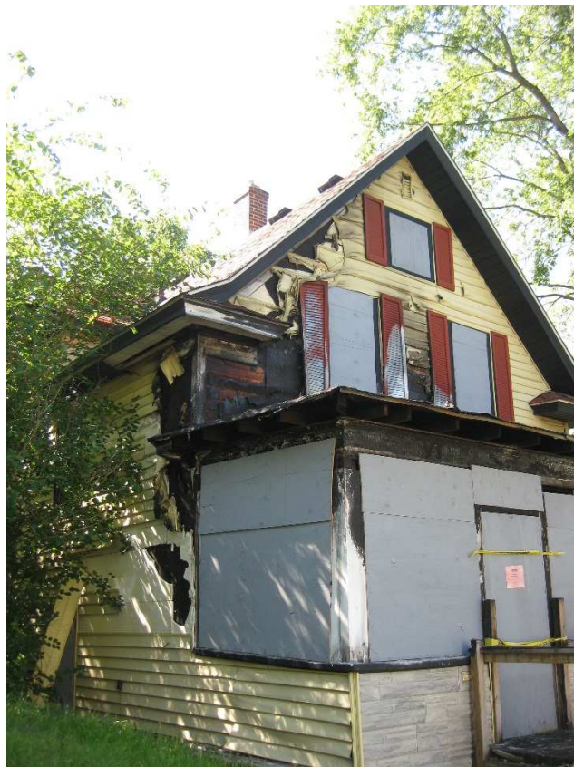
Picture 3 – Fire Damage, Northeast Elevation
