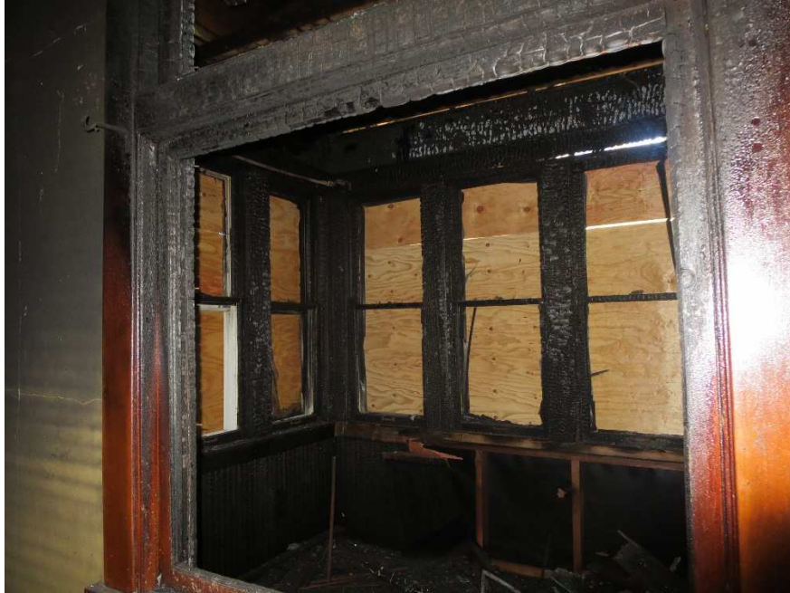
Picture 2 – Front Porch Fire Damage
