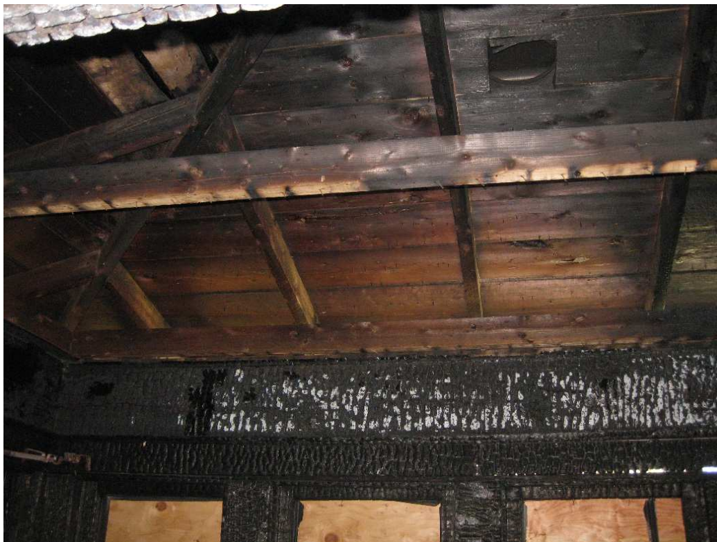
Picture 1 – Front Porch Fire Damage
