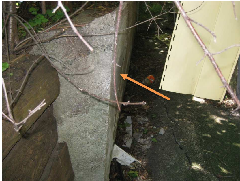
Picture 12 – Rotated Foundation Wall
