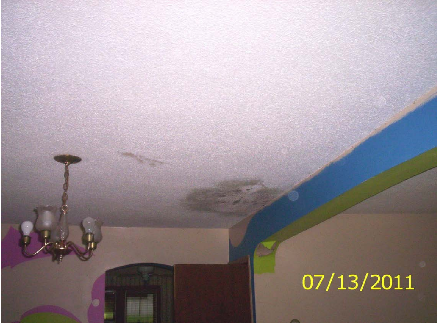
Water damaged ceiling, peeling paint, possibly mold
