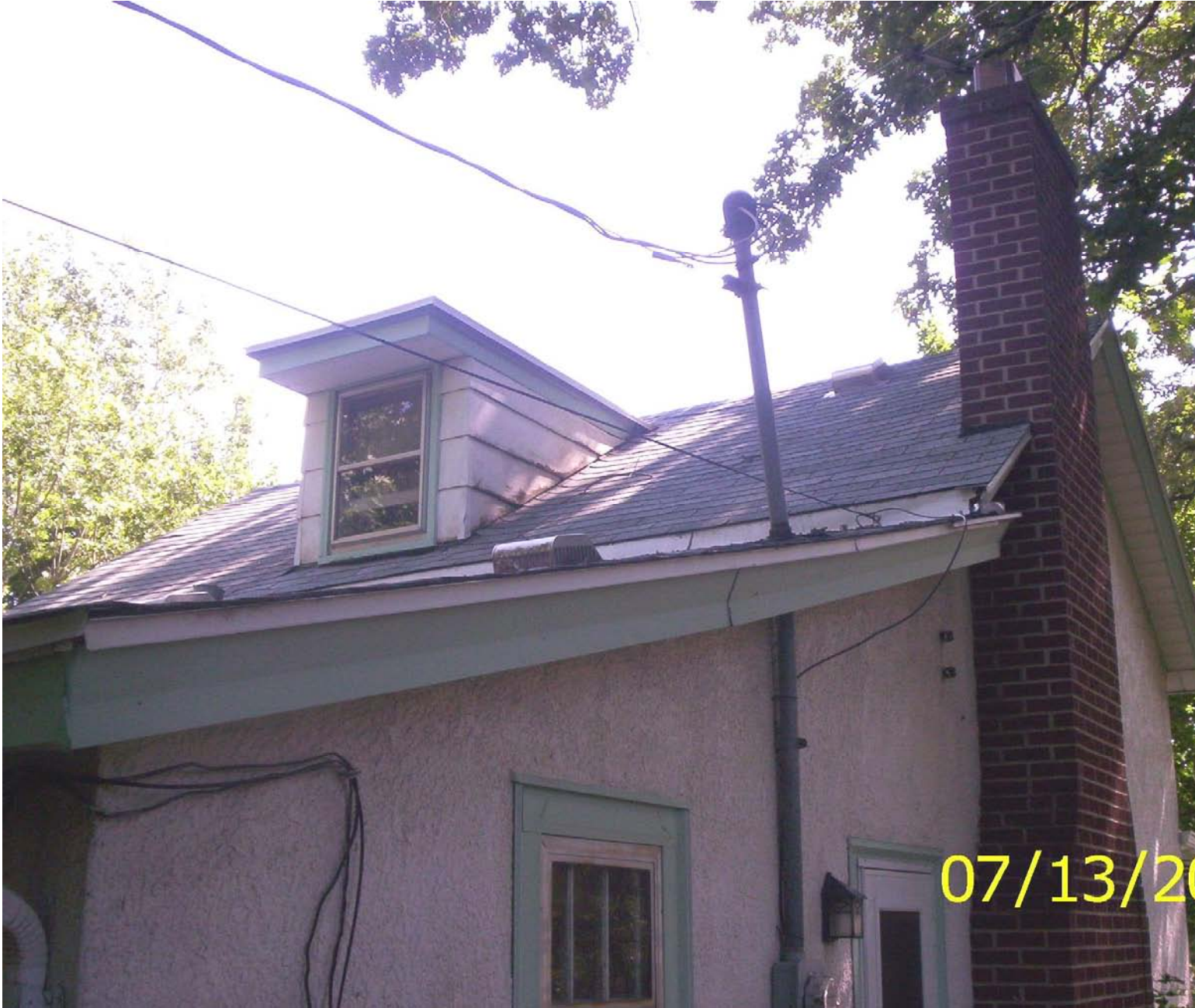
South and west face of the west side dormer, missing flashing, water damaged siding
