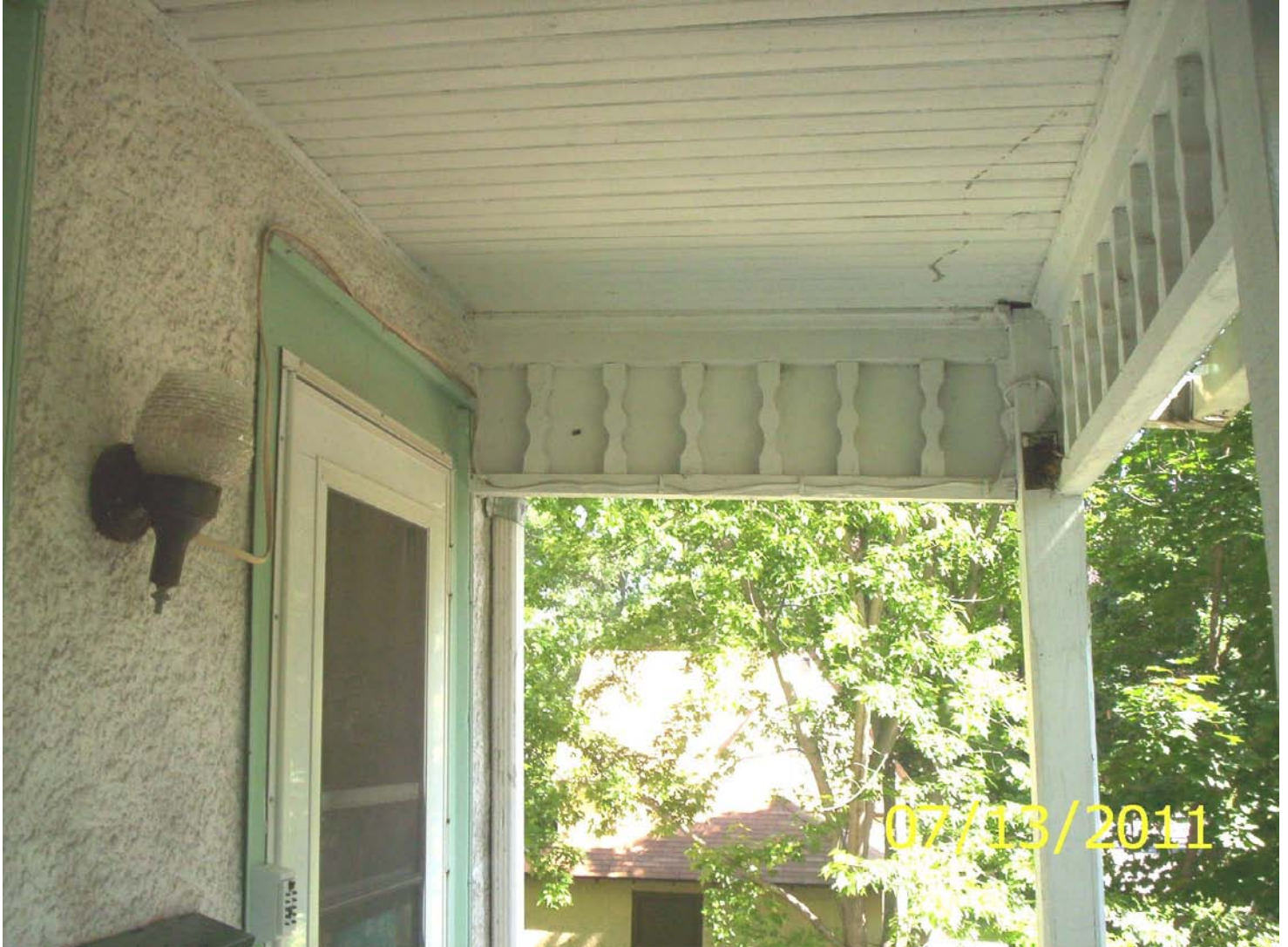
Unapproved exterior electrical wiring
