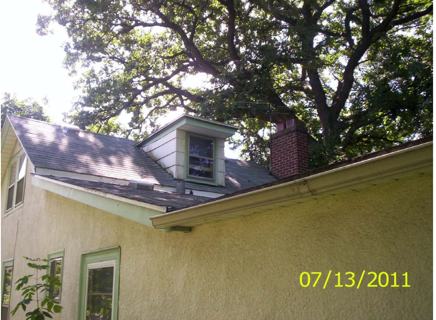
North and west face of the west side dormer, missing flashing, water damage siding
