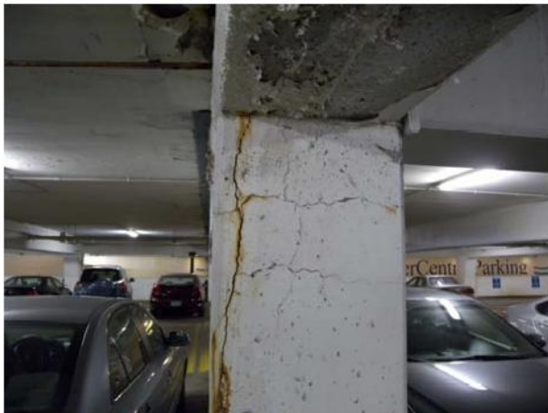
Cracking/delamination of column
