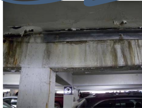
Concrete deterioration under angle
