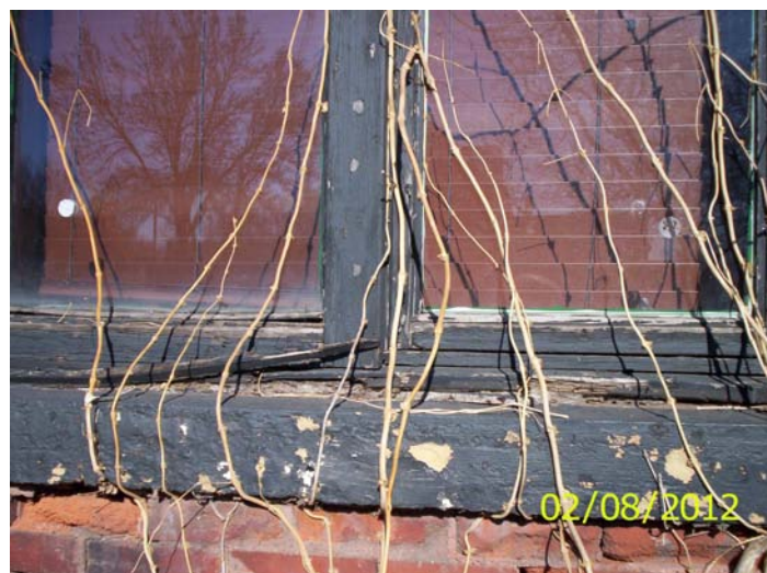
Deteriorated window frame, open wall
