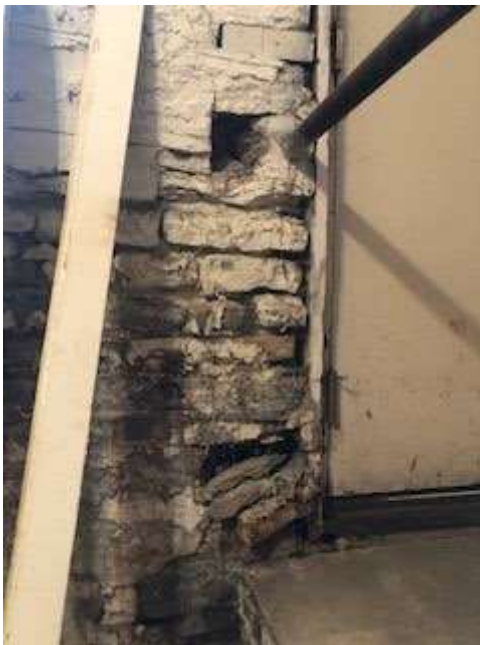
8: Settling and holes in foundation
