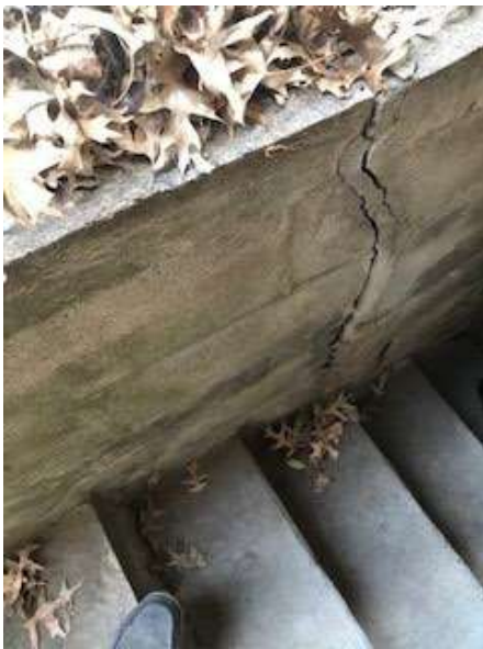
13: Cracks at concrete steps to Unit 5
