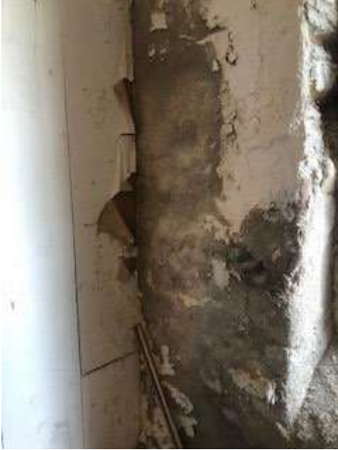
10: Flaking paint and worn foundation
