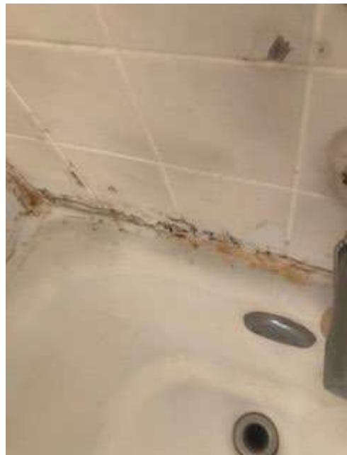
24: Mold and deterioration in unit shower
