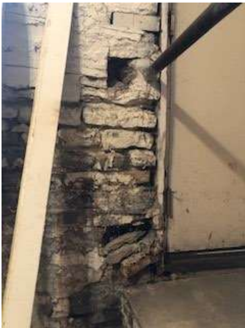
8: Settling and holes in foundation
