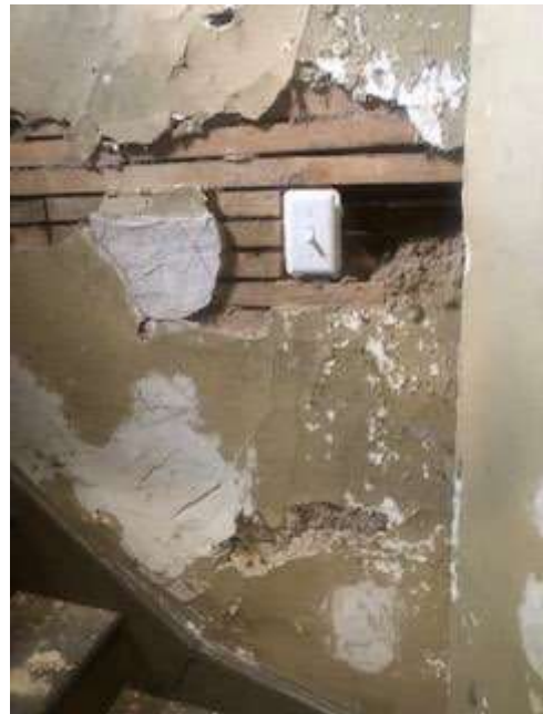
22: Wall deterioration at stairway
