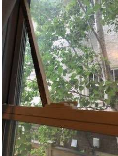
35: Tenant window held up by wooden post
