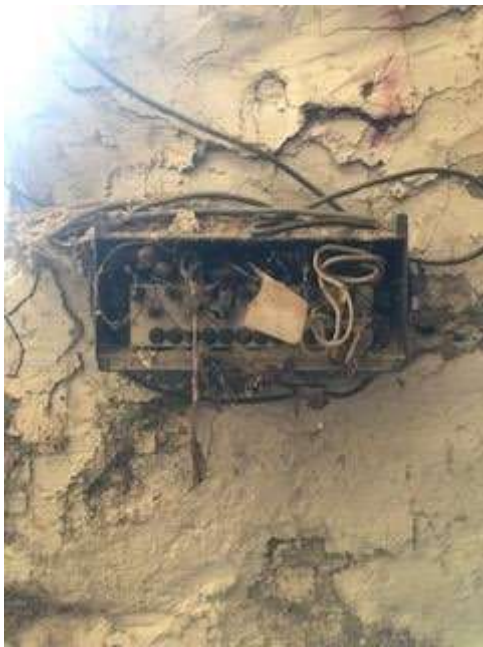
41: Electrical box missing cover
