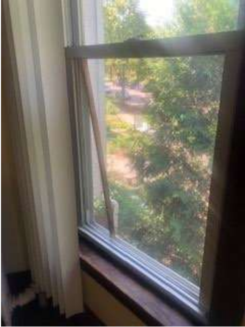
34: Tenant window held up by wooden post
