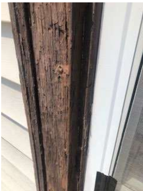
1: Rotting/peeling exterior trim
