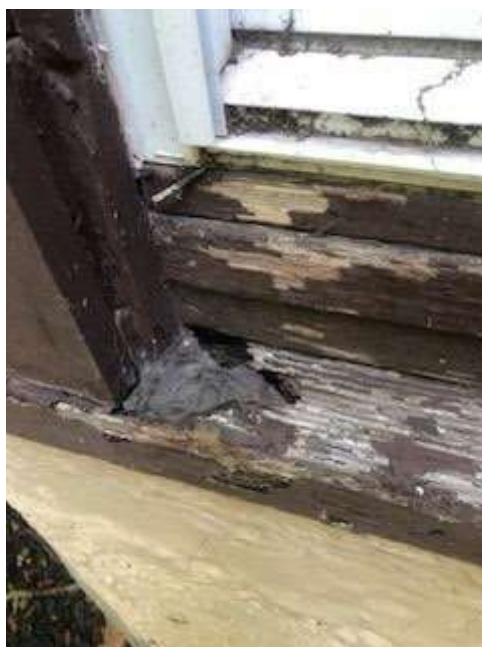
2: Rotting/peeling exterior trim and cavity
