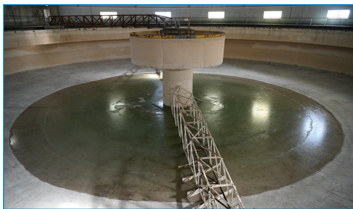
The large round clarifiers were both open for several weeks at the beginning of the year as part of annual plant maintenance efforts. This is clarifier two as seen on Jan. 21 after cleaning was completed.
