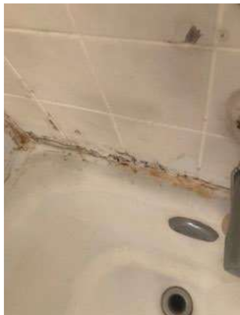
24: Mold and deterioration in unit shower
