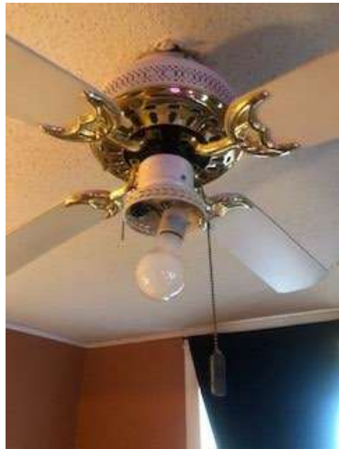
44: Wobbly fan in tenant unit w/o cover
