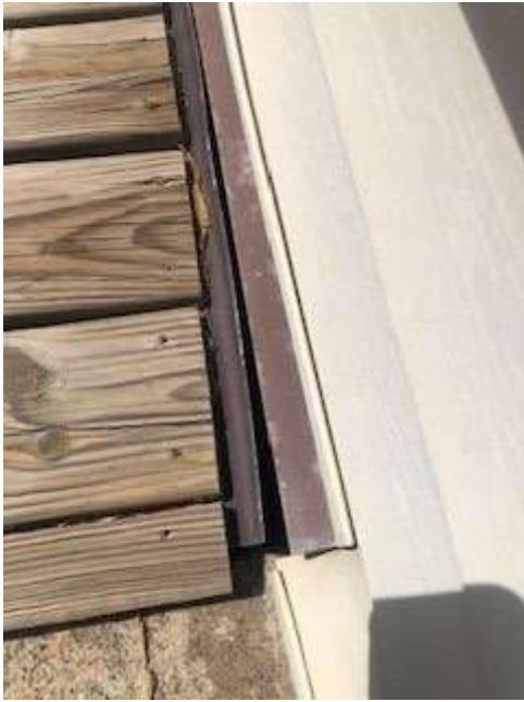
5: Wooden balcony separating from siding
