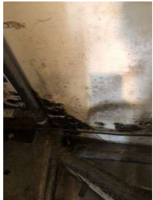
20: Mold at laundry room walls
