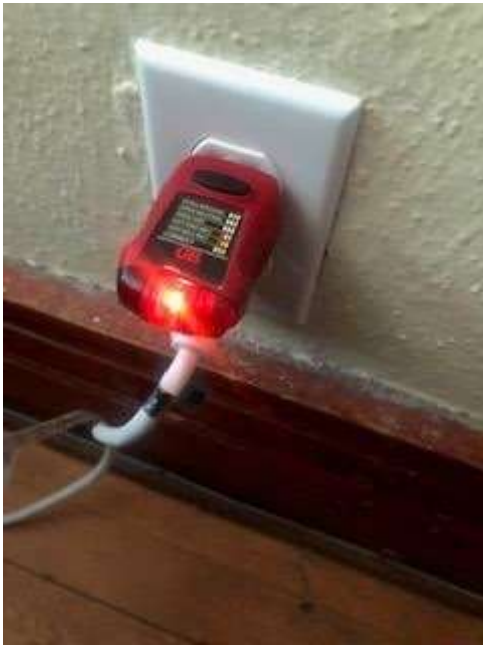
43: Testing unit showing open ground outlet
