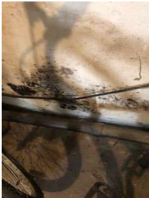
19: Mold at laundry room walls
