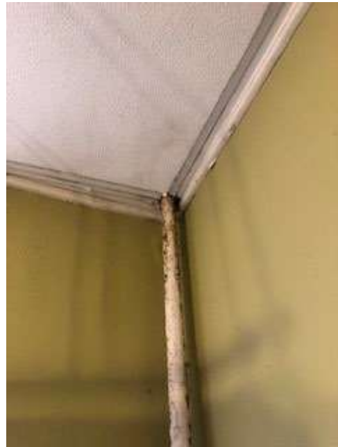
26: Mold/rust on exposed pipe
