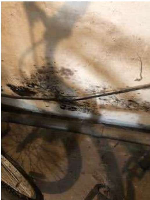
19: Mold at laundry room walls
