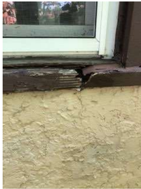
4: Rotting/peeling exterior trim and cavity
