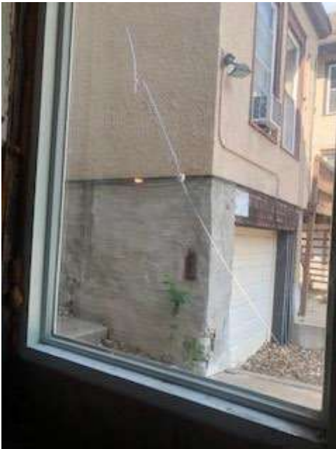
36: Cracked window in laundry room
