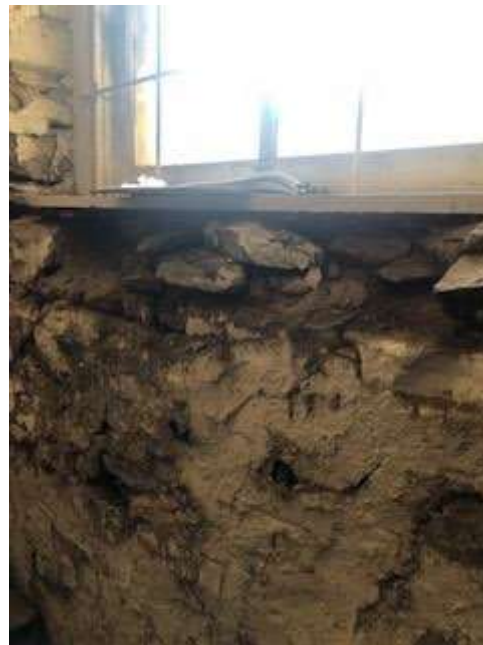
9: Deteriorating foundation at basement window
