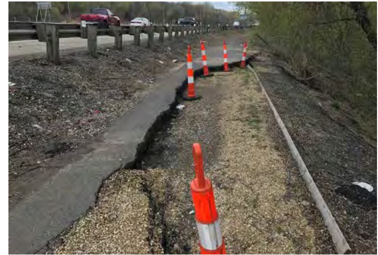
Segment 1 slope failure along southbound Hwy 61.
