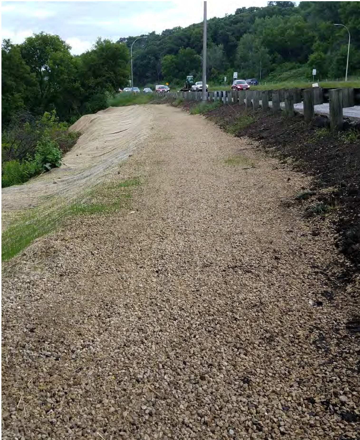
Segment 1: Looking north along Hwy 61. Aggregate base in place as a temporary measure where the slope failed due to erosion.
