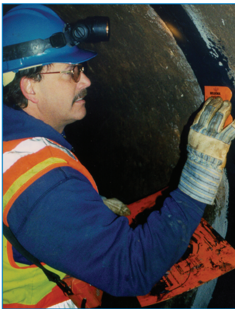
Rick Svoboda repairs a joint on a conduit in the early 2000s.
