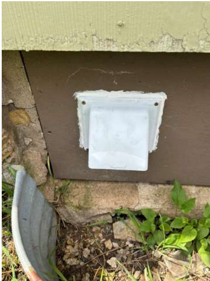
Picture of dryer vent as requested
