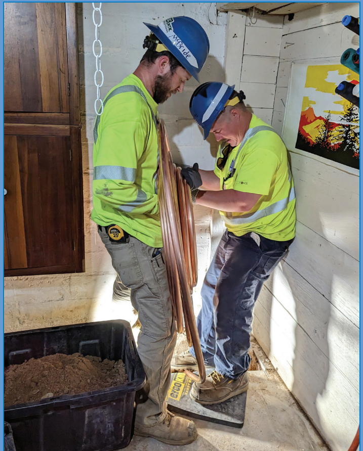
Left, Nick McBride, water system worker II, and Samuel Bartz, water utility worker I, feed copper pipe through the basement of a day care on Jessie Street on May 25.
