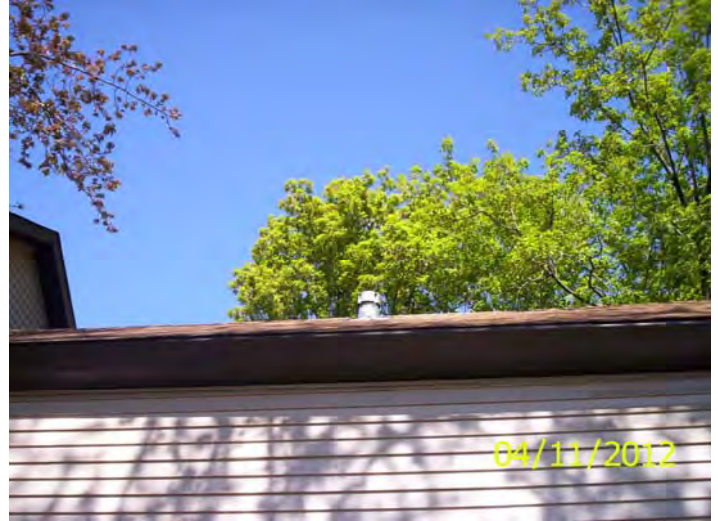
Gas fired appliance vent wrapped in what appears to be aluminum foil – possible moisture leak
