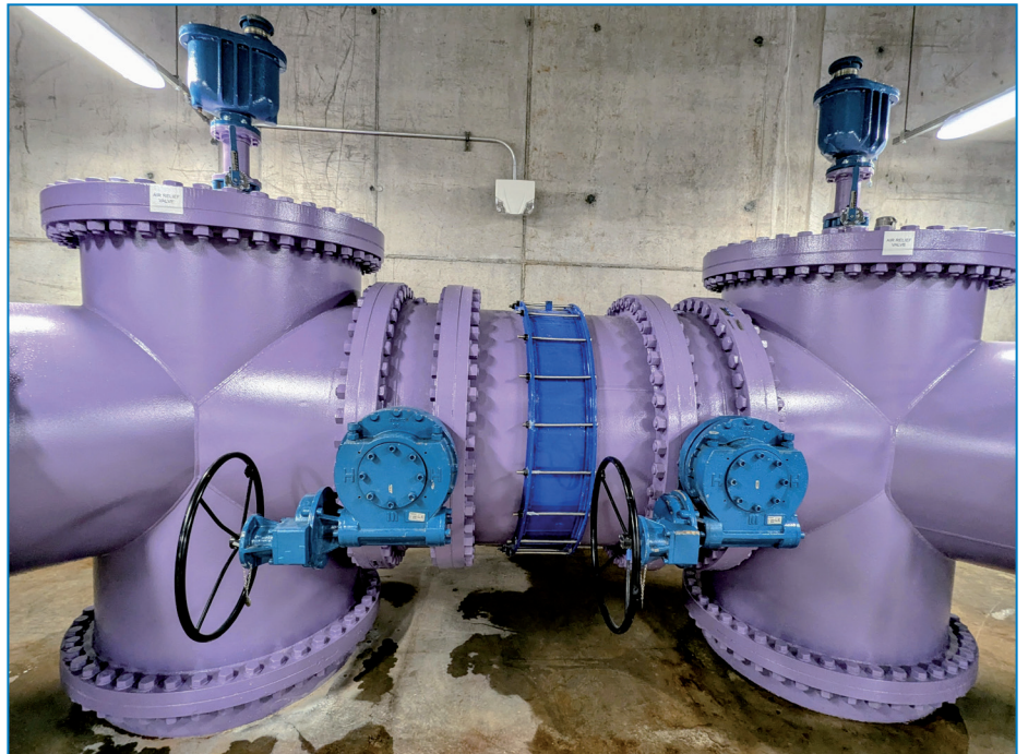
Newly painted 72-inch pipes bring raw water into the treatment plant.
