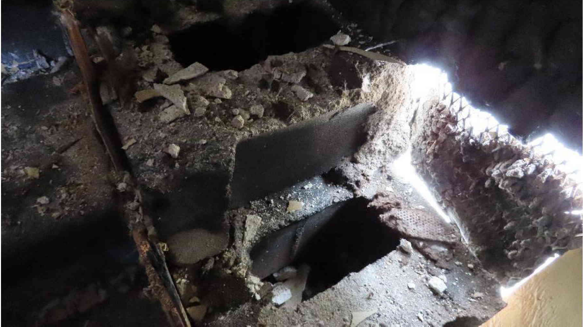
Photograph 15: Soot stained CMU block.
