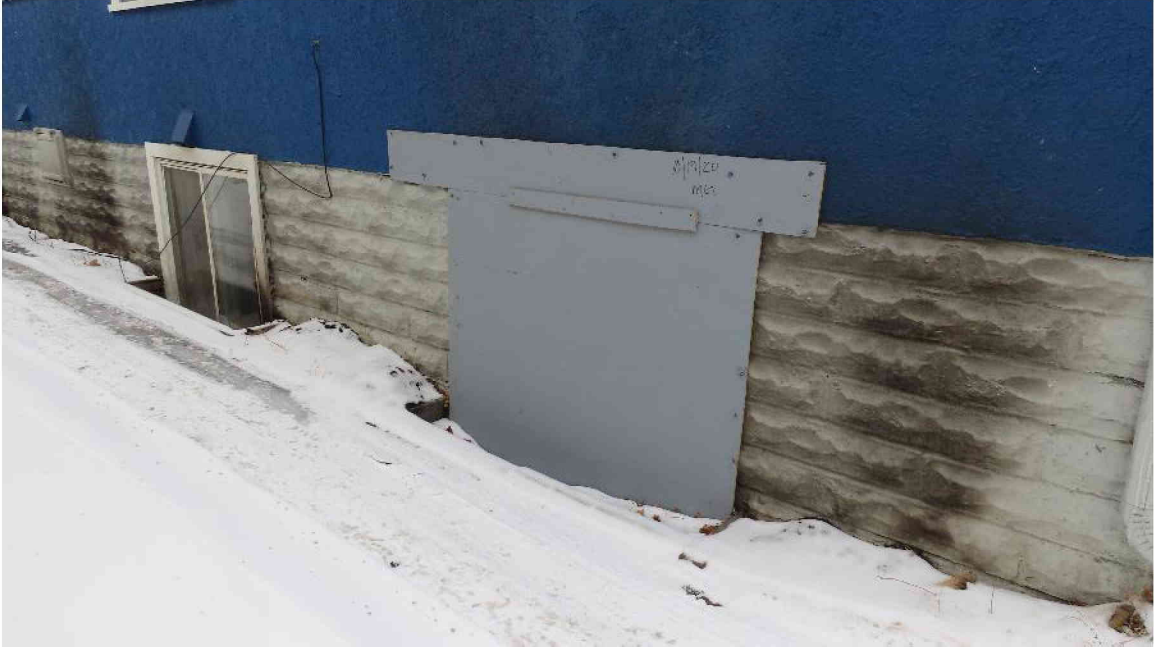
Photograph 19: Soot stained exterior walls at boarded up window on the north wall.
