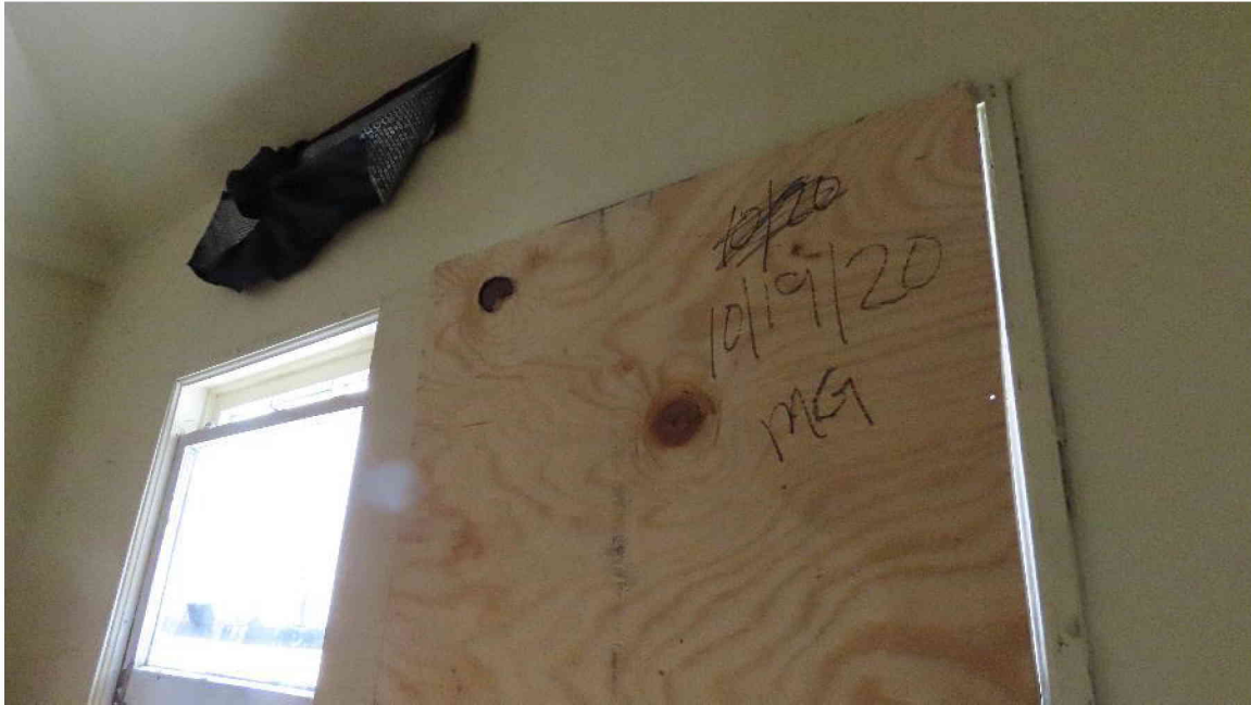
Photograph 17: Boarded up north window in the upper-level bedroom.
