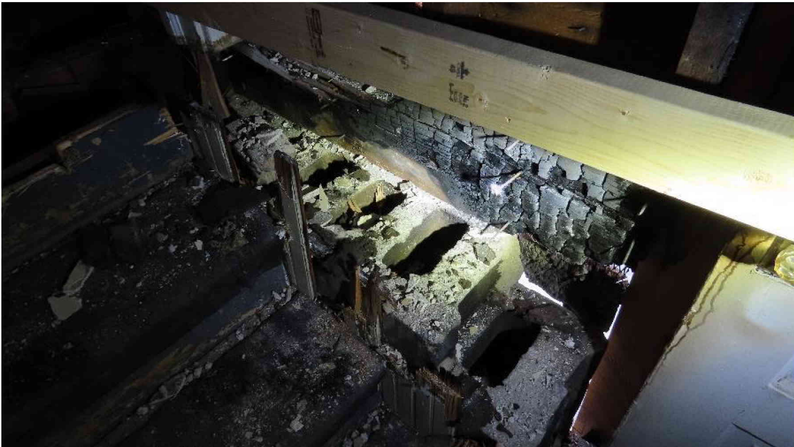
Photograph 14: Charred wall sheathing at the north door.
