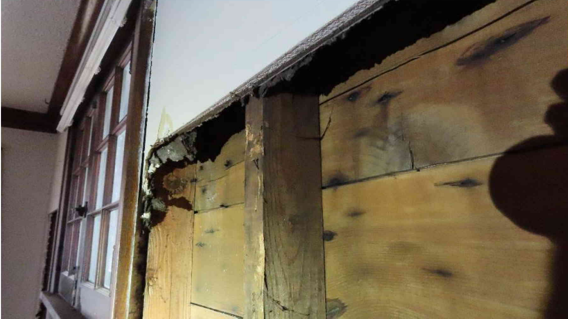
Photograph 9: Soot stained wall framing.
