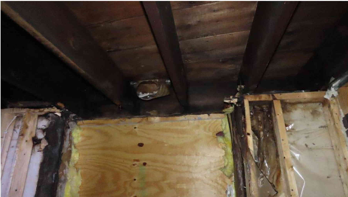
Photograph 6: Window header is missing.
