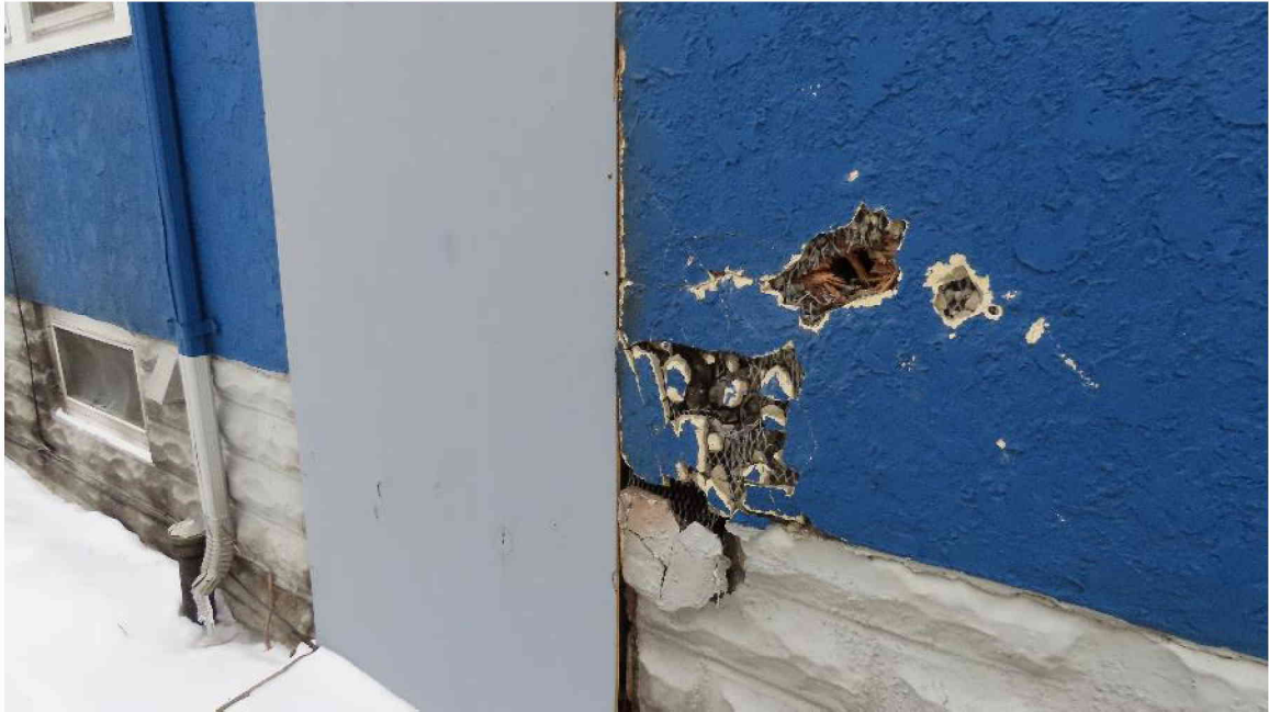
Photograph 21: Holes in stucco at the boarded-up door.
