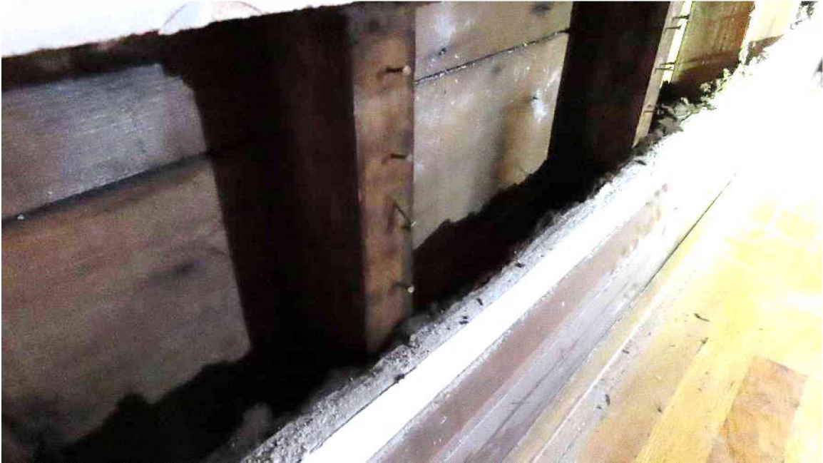
Photograph 11: Soot stained wall framing.
