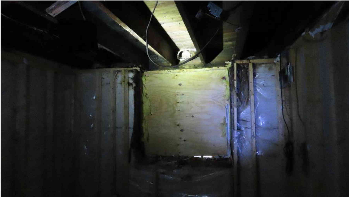
Photograph 5: Boarded up window in the northwest basement bedroom.
