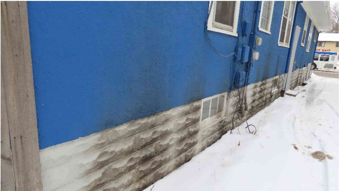
Photograph 20: Soot stains on the north wall.
