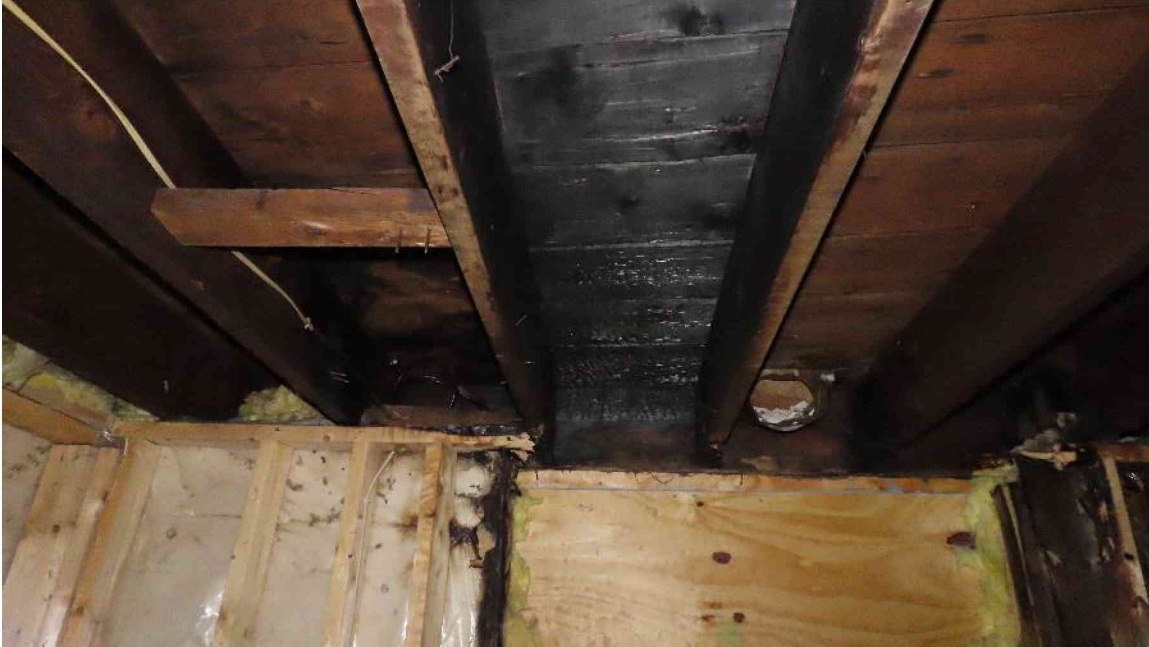
Photograph 7: Charred floor joists and decking at the northwest basement bedroom.
