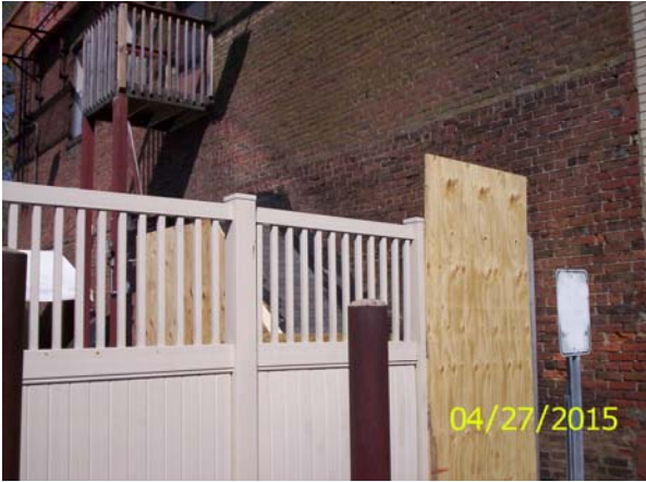
Patio area burned
