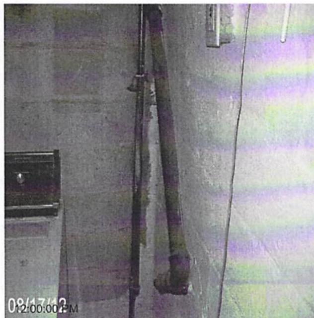
Date Completed: before: bond water meter
