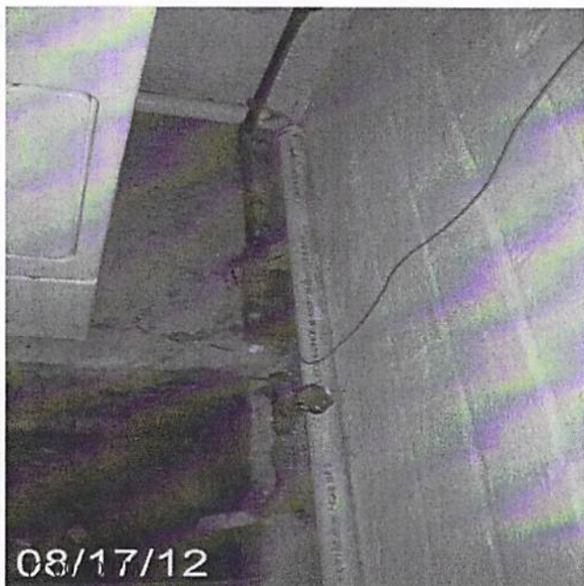
Date Completed: before: bond water meter
