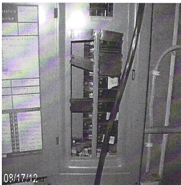
Date Completed: before: circuit breaker amp
