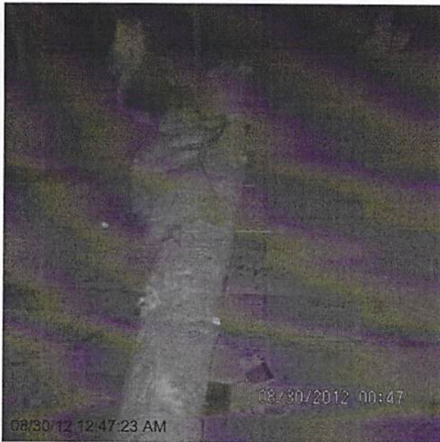
Date Completed: 09/03/2012 miscellaneous-cover 3 holes in floor in attic, eac
