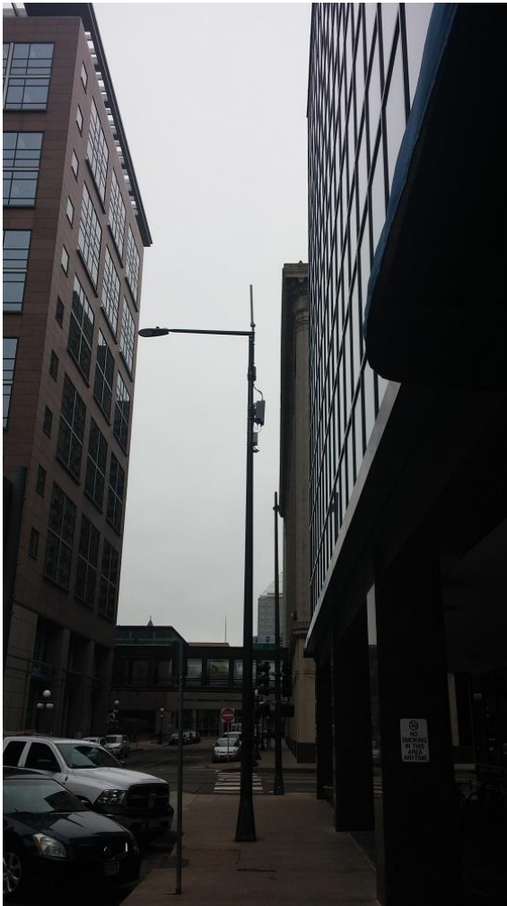
Sample Small Cell Installation in Saint Paul
