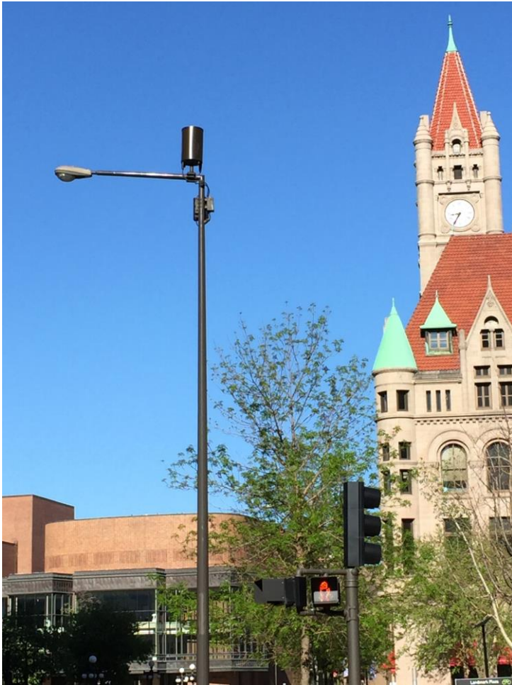
Sample Small Cell Installation in Saint Paul
