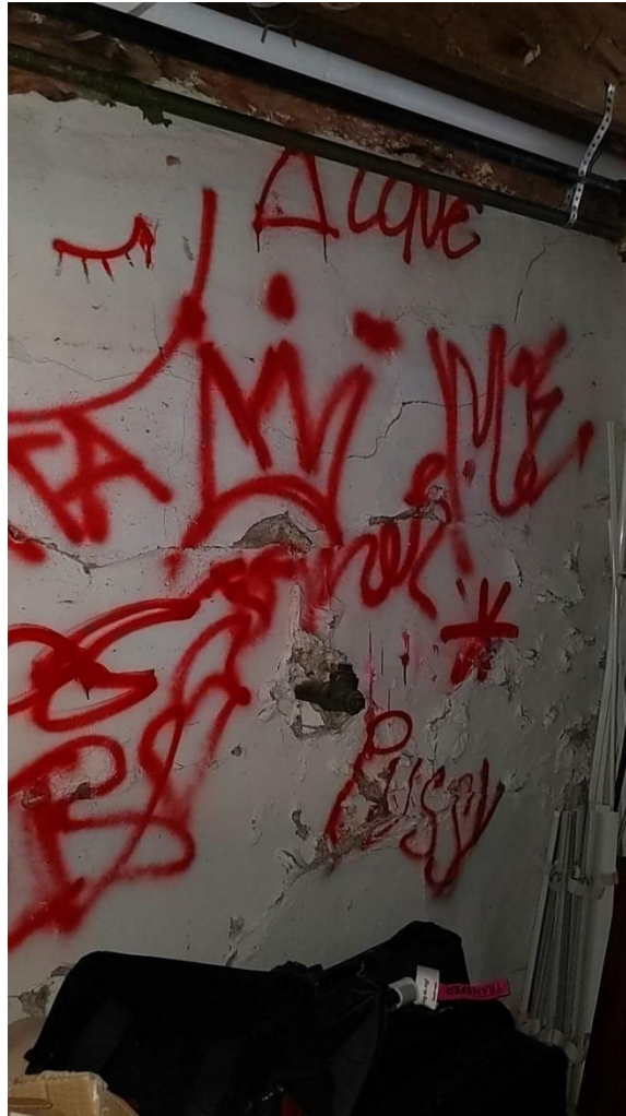
Figure 1: Parge Coating at End of Life (Delaminated)
