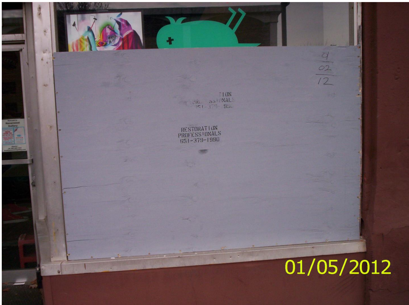
Window secured by SPPD
