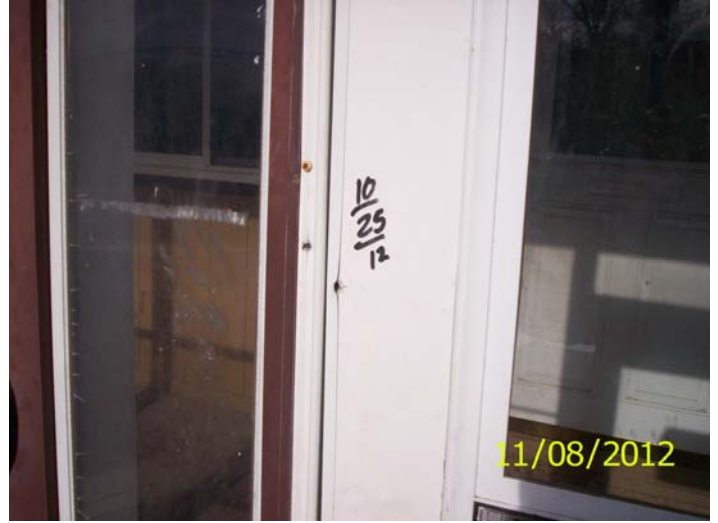
Date of secure, front storm door
