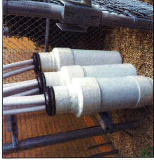
1 CONDUIT AT SHELTER PHOTO SCALE: NONE
