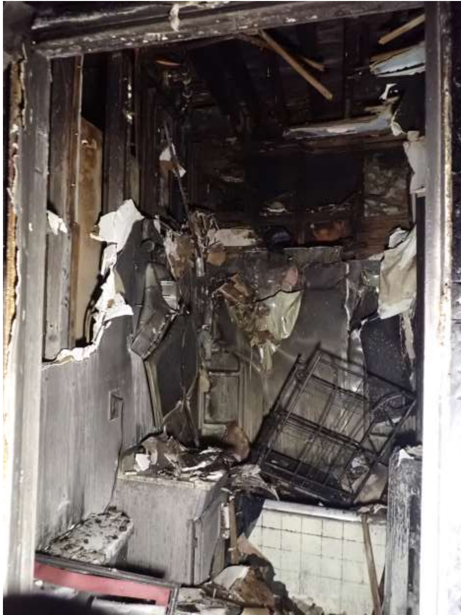
326 Charles Ave – Fire photos sent on 7/11/23
