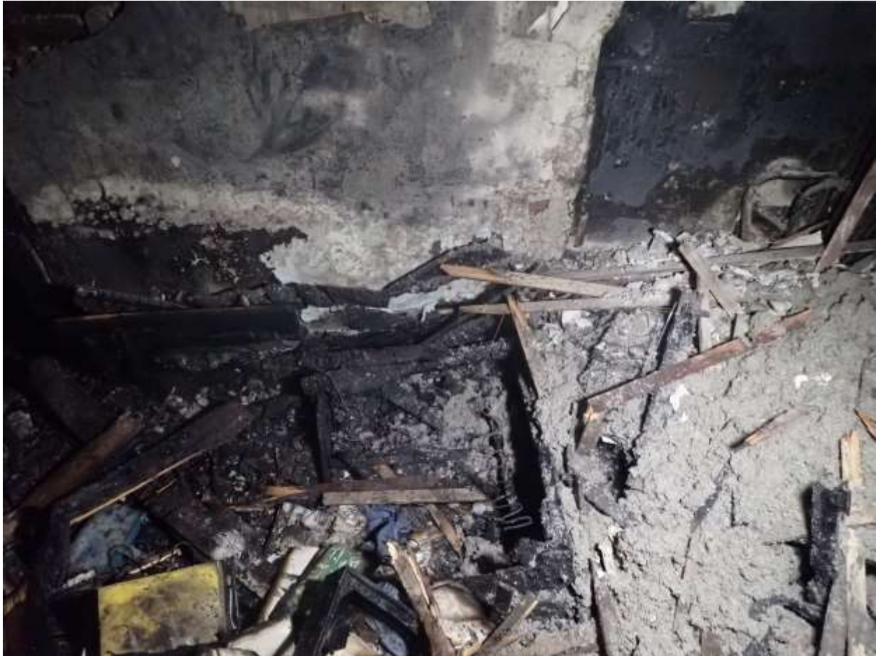
326 Charles Ave – Fire photos sent on 7/11/23
