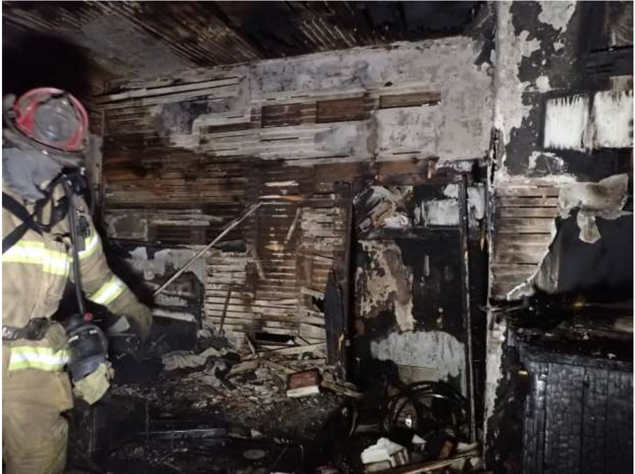
326 Charles Ave – Fire photos sent on 7/11/23
