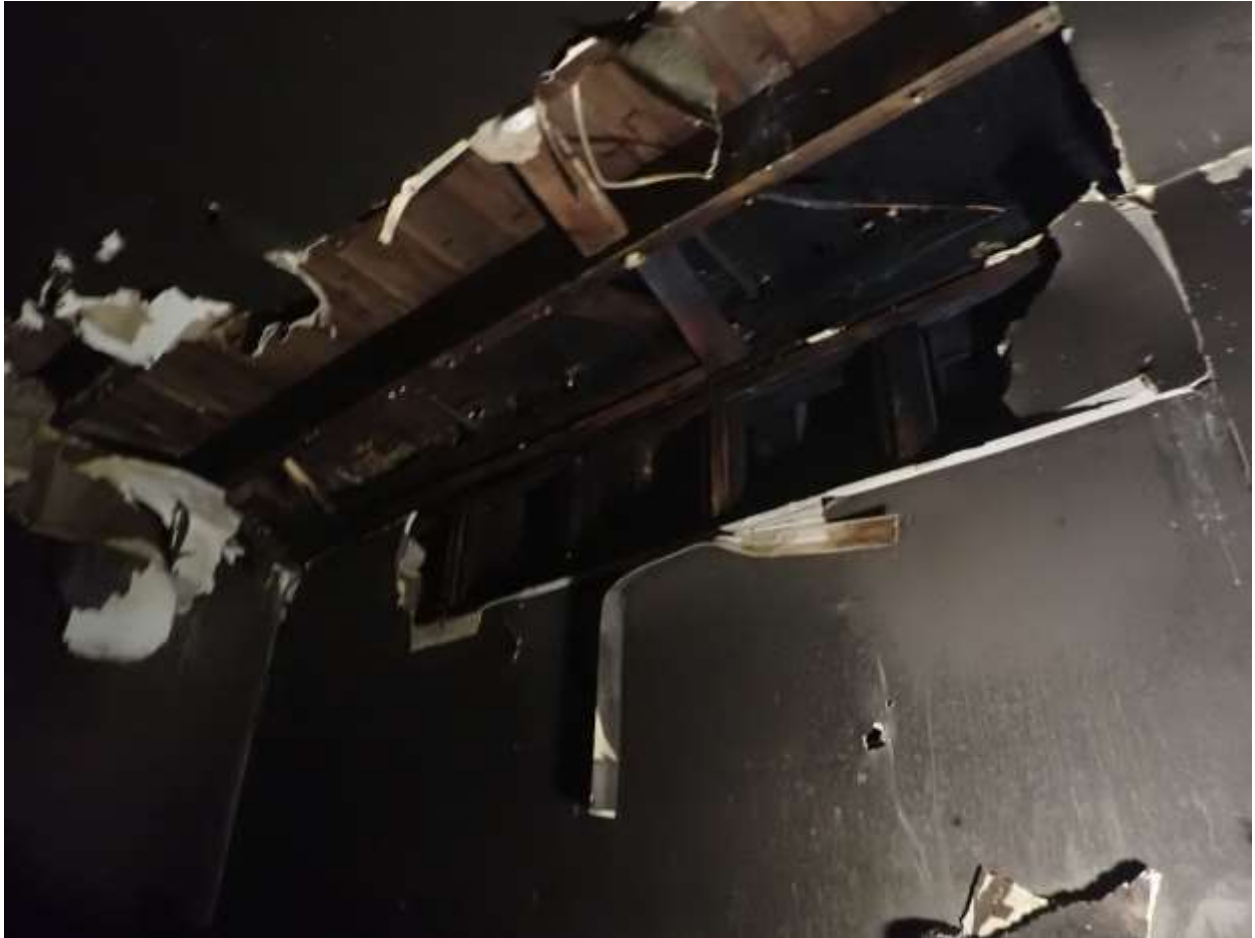
326 Charles Ave – Fire photos sent on 7/11/23
