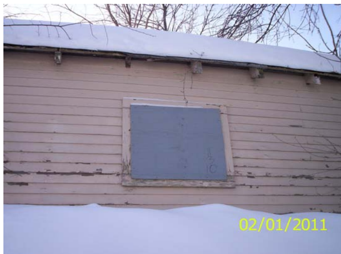
Garage securing by City
