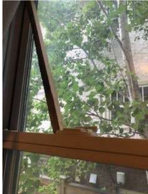
35: Tenant window held up by wooden post
