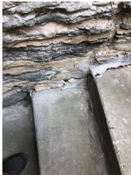
14: Mortar gaps at concrete steps to Unit 5
