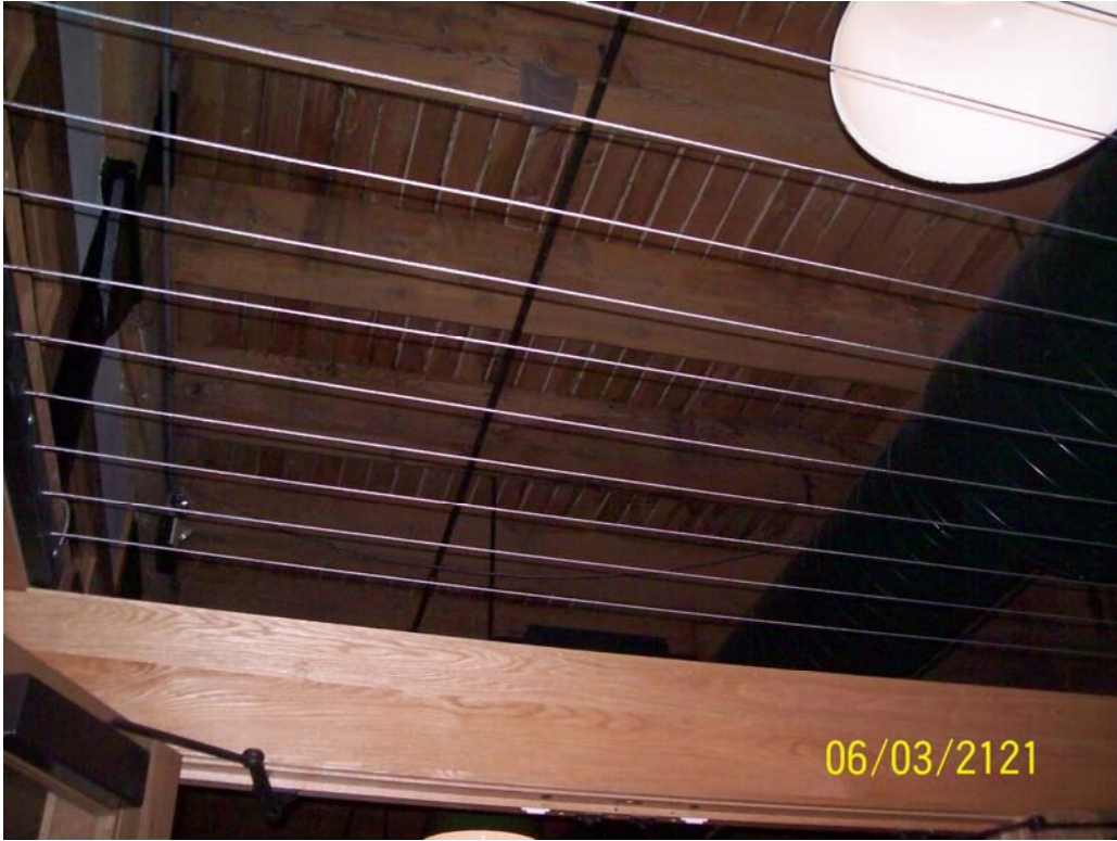
Above egress door with slide bolts.
