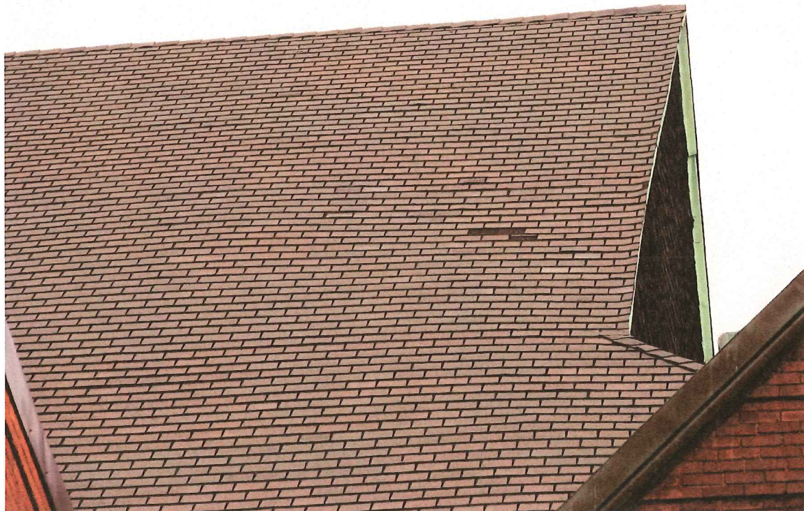
Figure 7 Detail of current portion of south side eastern end of main roof showing missing shingles 7/27/15
