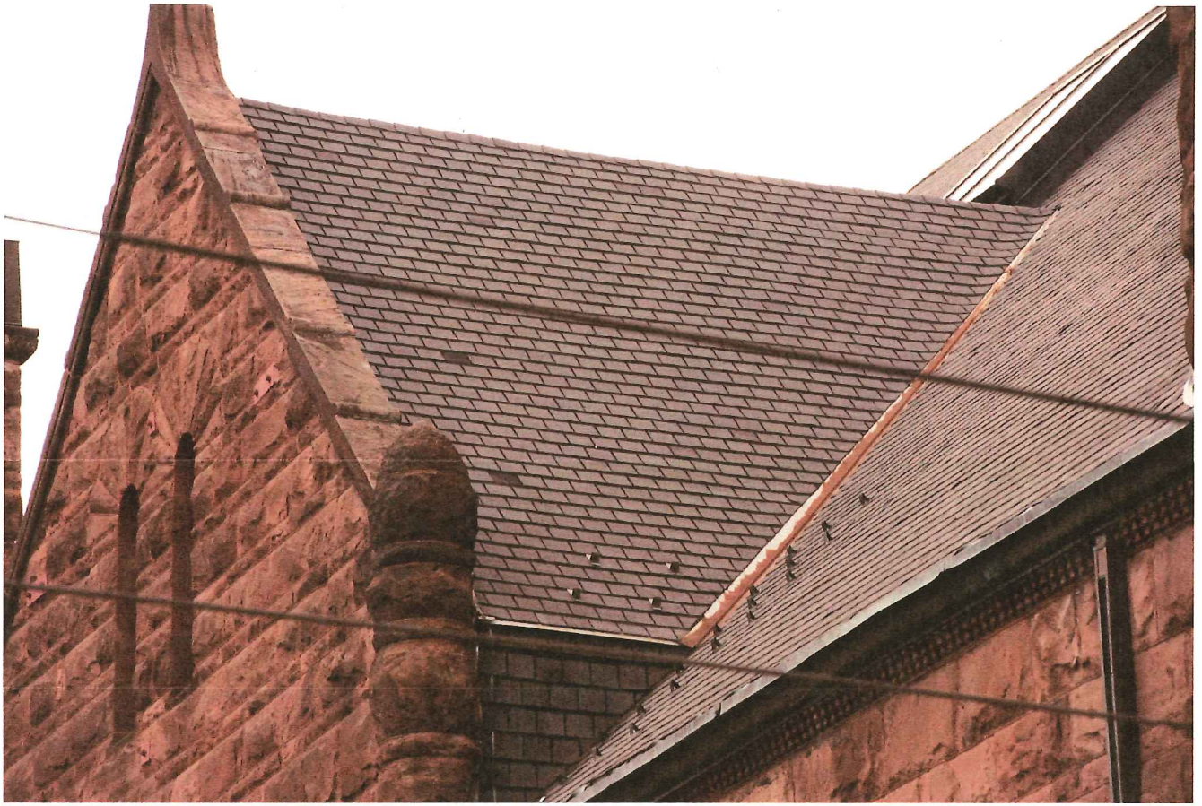
Figure 12 Detail view of gable of northeast corner showing missing shingles 7/27/15
