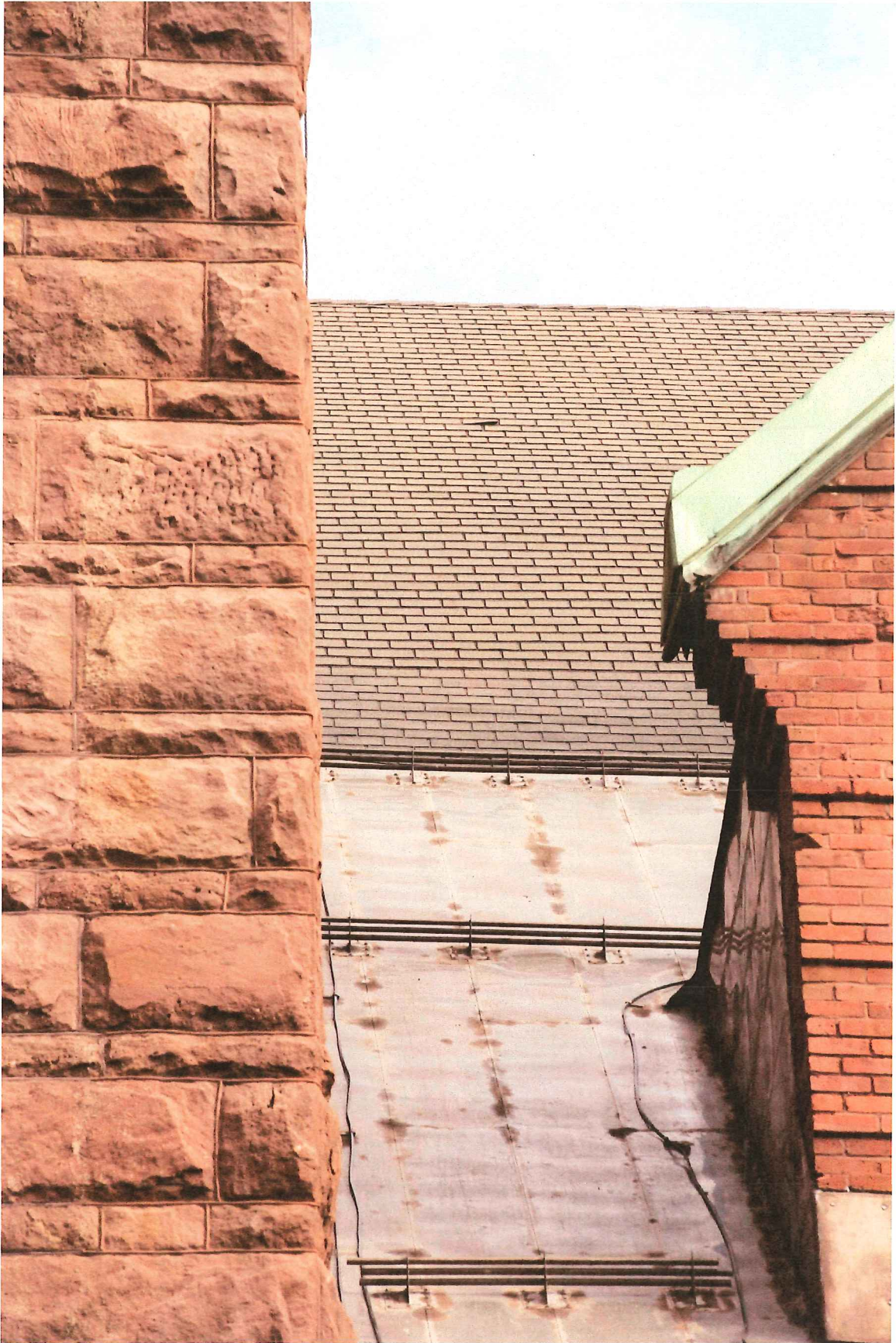
Figure 8 Detail view of south side main roof by bell tower showing missing shingles 7/27/15
