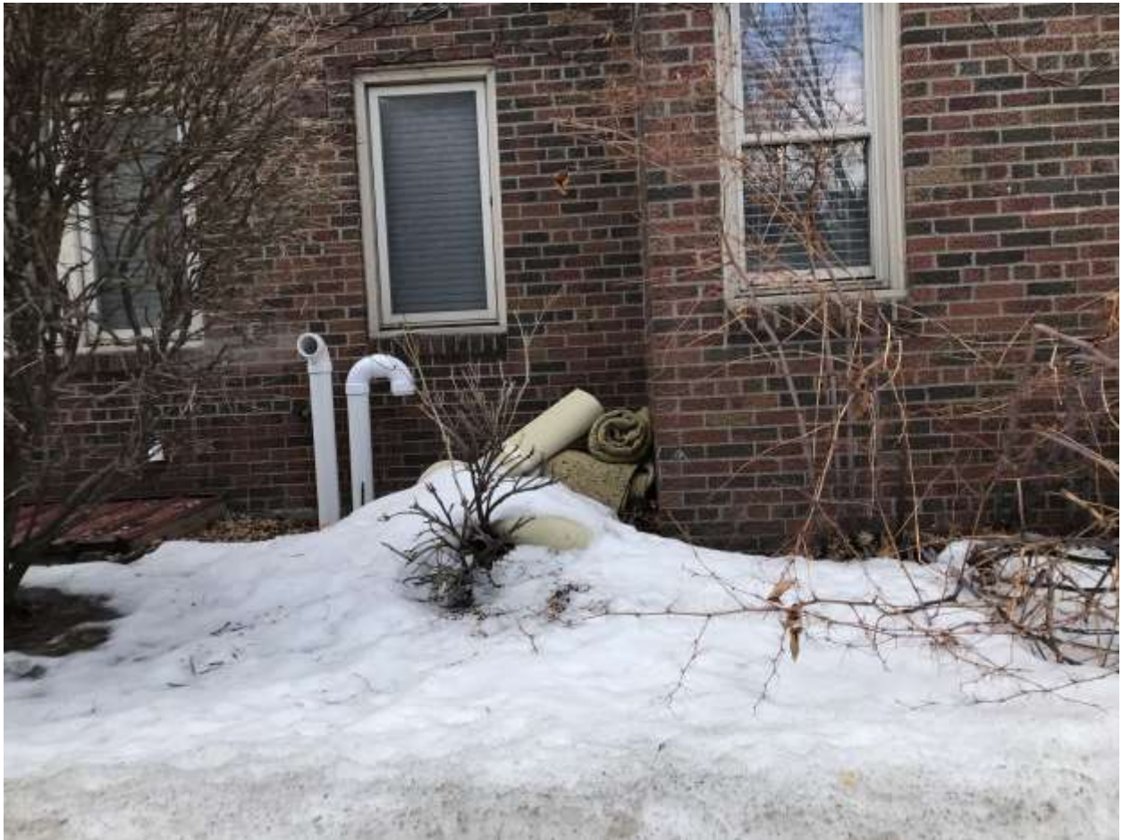
503 Cleveland Ave S. Taken 3/20/19
