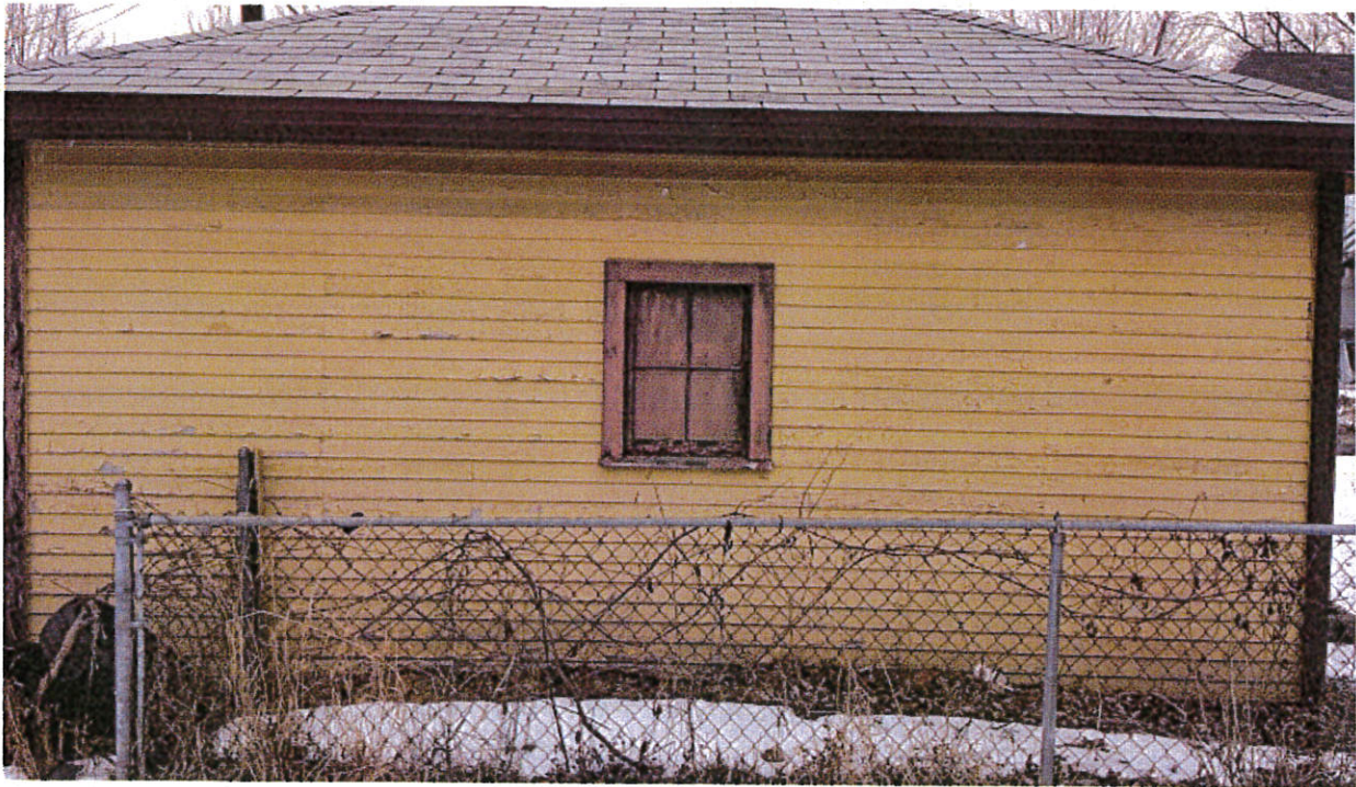
Image - picture of wall where paint is starting to deteriorate:
